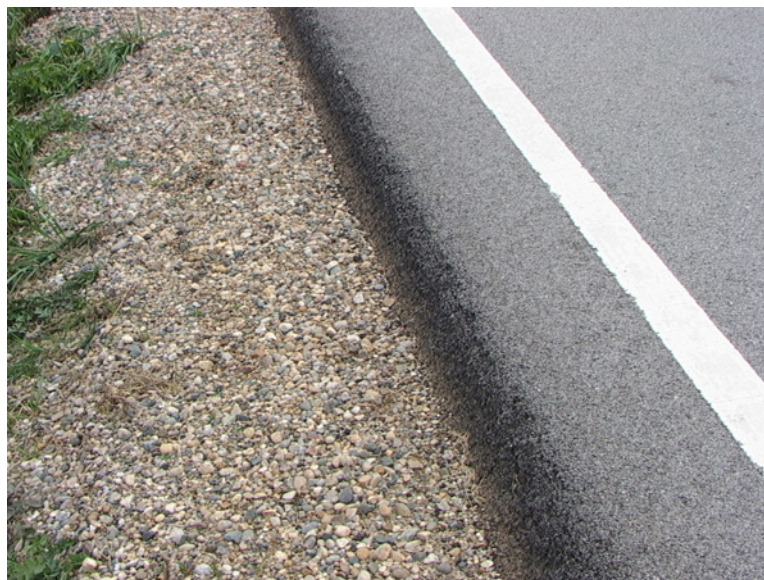
Figure 3. Exposed Safety Edge
