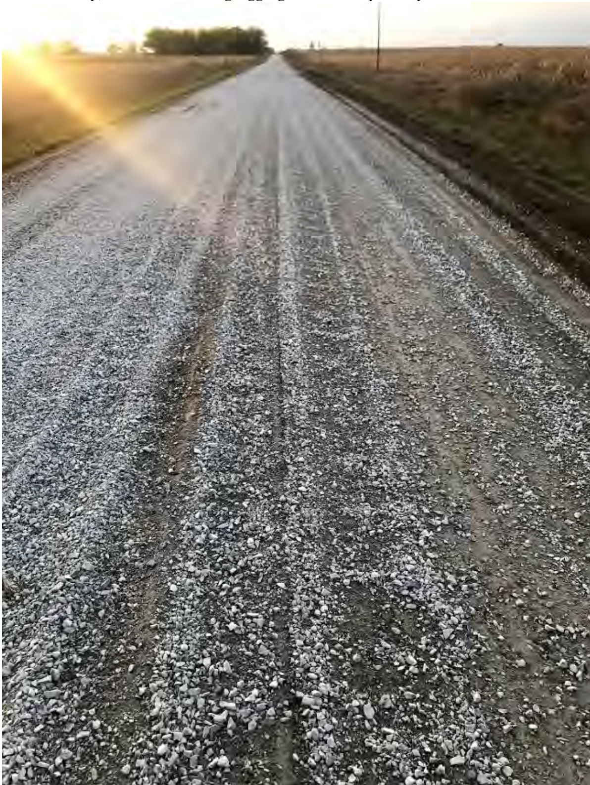
Appendix A – Figure 14. Clay Slurry section in Boone County, one day after construction, November 2019
