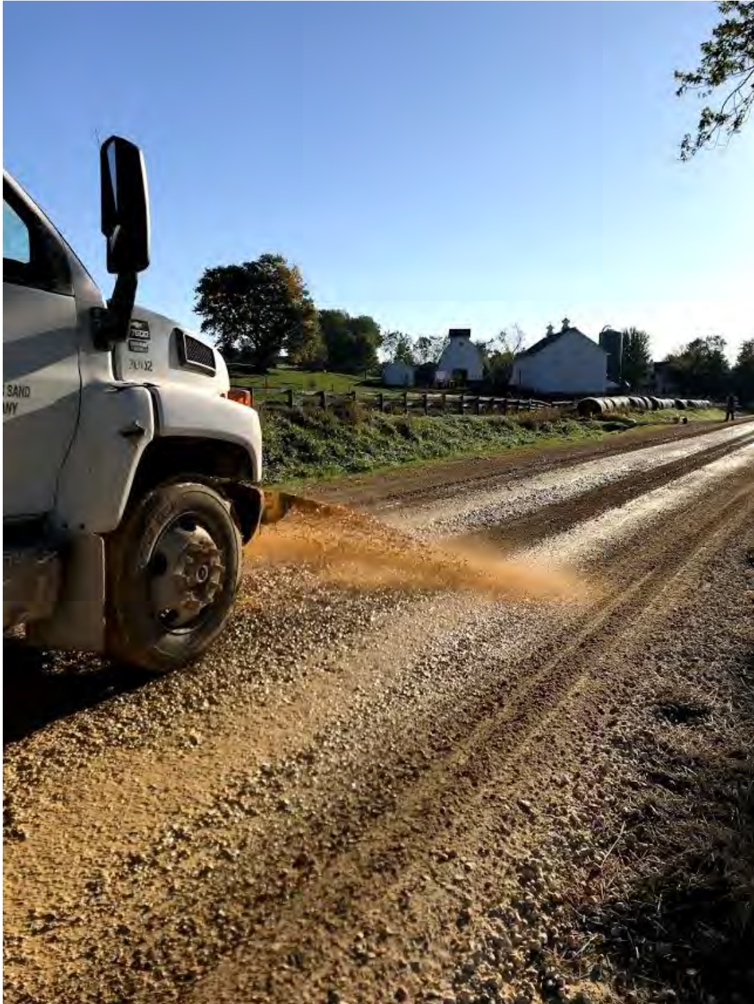
Appendix A – Figure 1. Spray tank for Clay Slurry section, Jones County, November 2019
