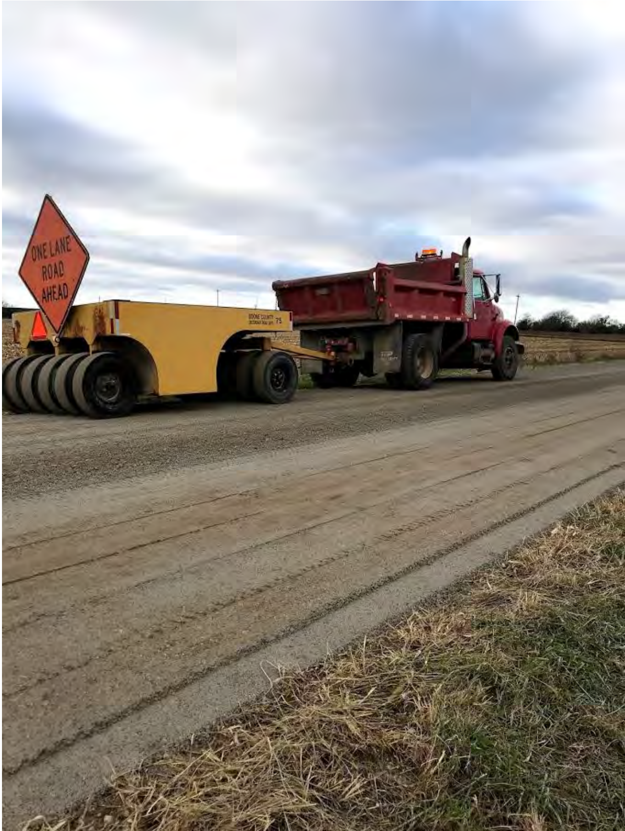
Appendix A – Figure 4. Roller used to compact the shaped surfaces in Boone County
