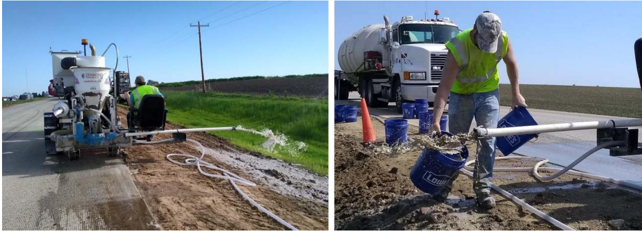
Figure 2: Direct Discharge CGR Collection (Site CGR-3 Shown)
