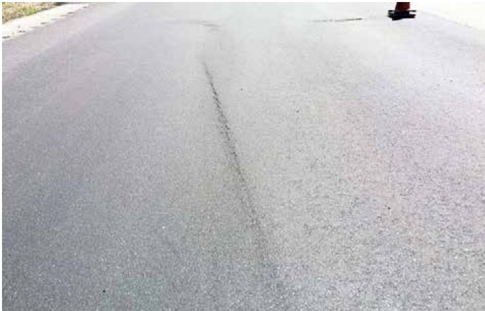
Figure 3 Slippage Failures of Section N7 After Repaving
