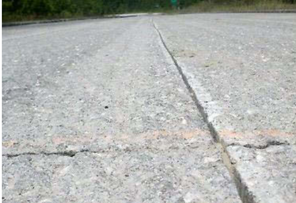
Figure 1 Deep Saw Cuts to Simulate Pavement Cracks
