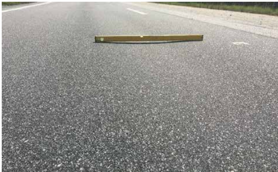
Figure 8 Rutting in Section N12
