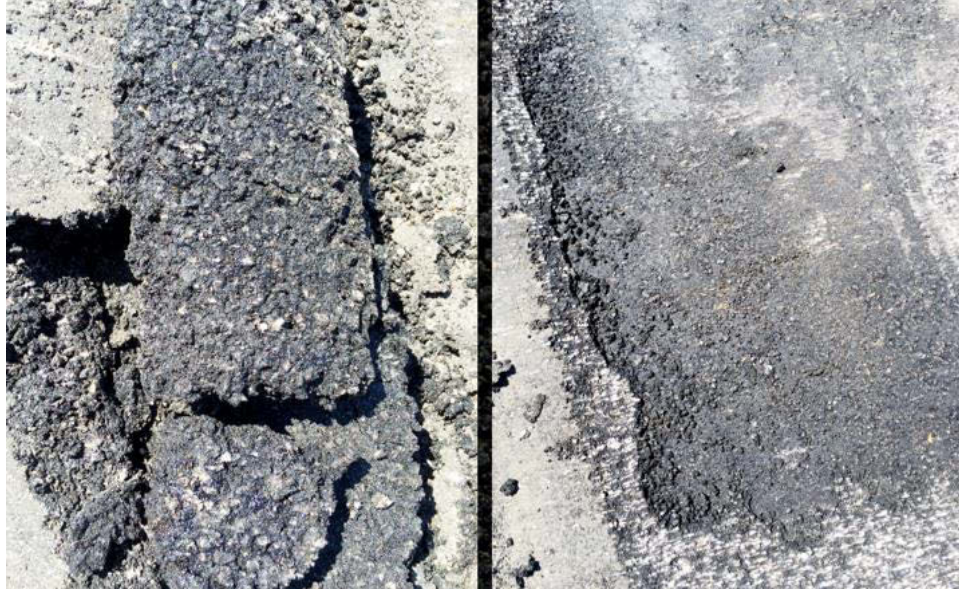
Figure 4 Interface Between Layers in Failure Area
