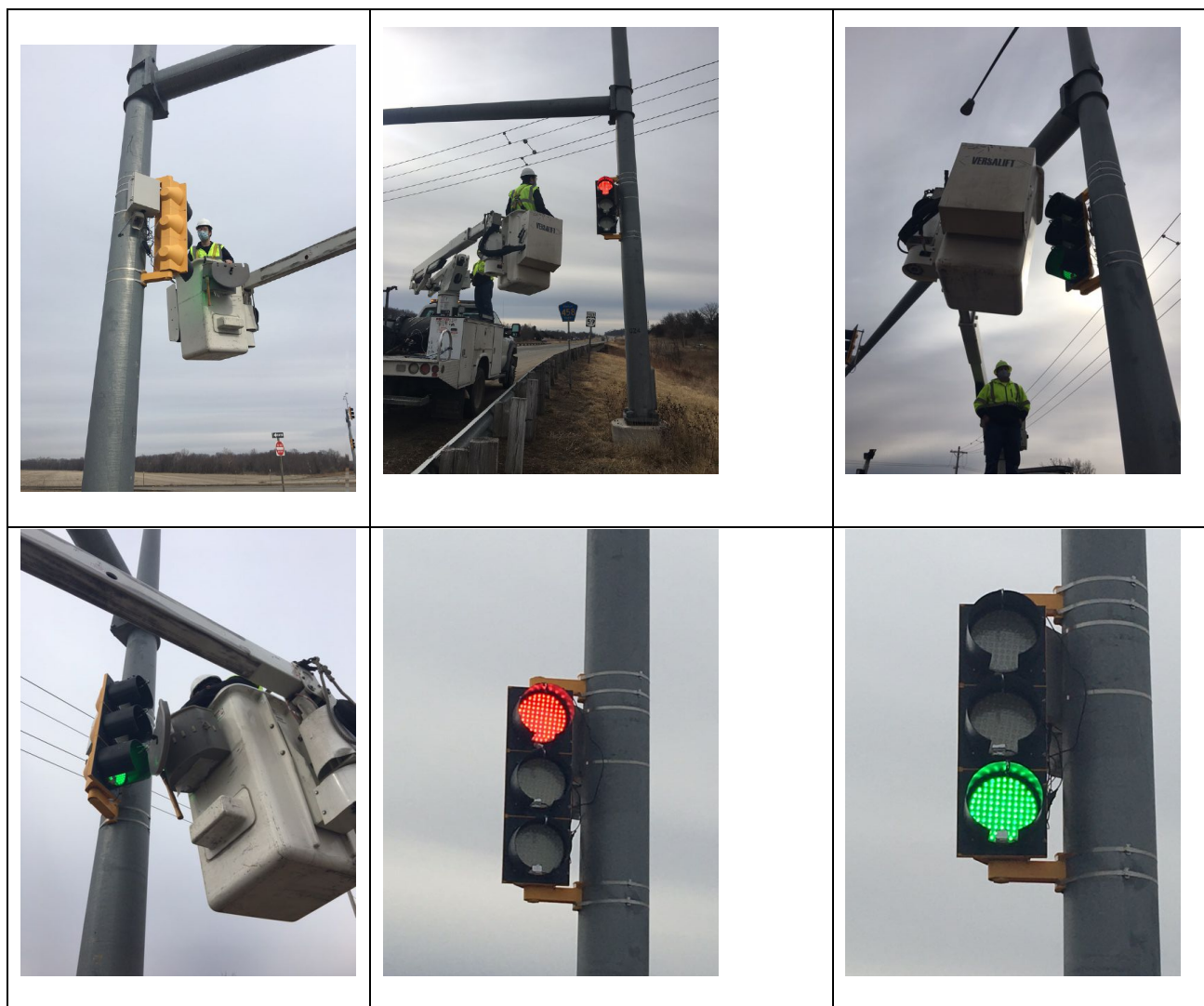
Figure 5 We stopped at the Lawrence field test site on Feb 25 th , with the Lawrence signal crew, to fix two problems related to the data collection and performance remote monitoring system (not part of the self-de-icing signal lights). We replaced the problematic cable cameras which failed after being exposed to the environment in the past two years. We also fixed the loose mounting of temperature sensors.
