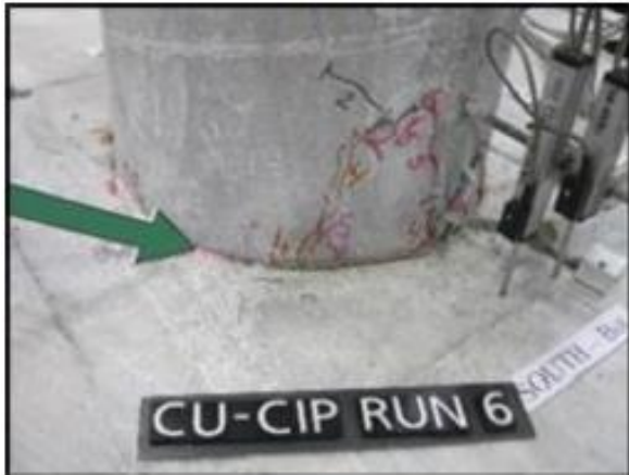
Fig. 3- Damage after 3.5 time design earthquake
