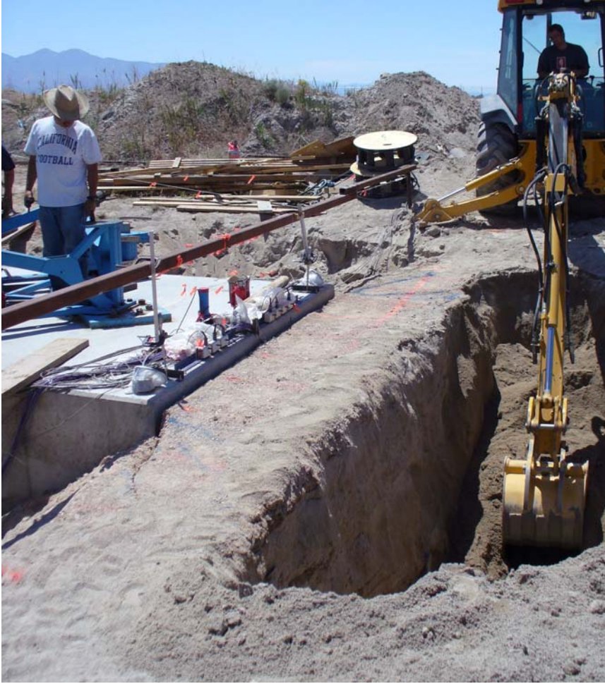
Fig. 2. 0.9m wide granular backfill zone adjacent to test cap during removal of loose sand backfill
