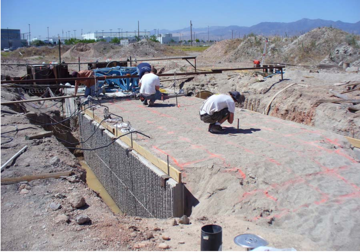
Fig 3. Looking south at MSE wall section with test pile cap and eccentric-mass shaker in background
