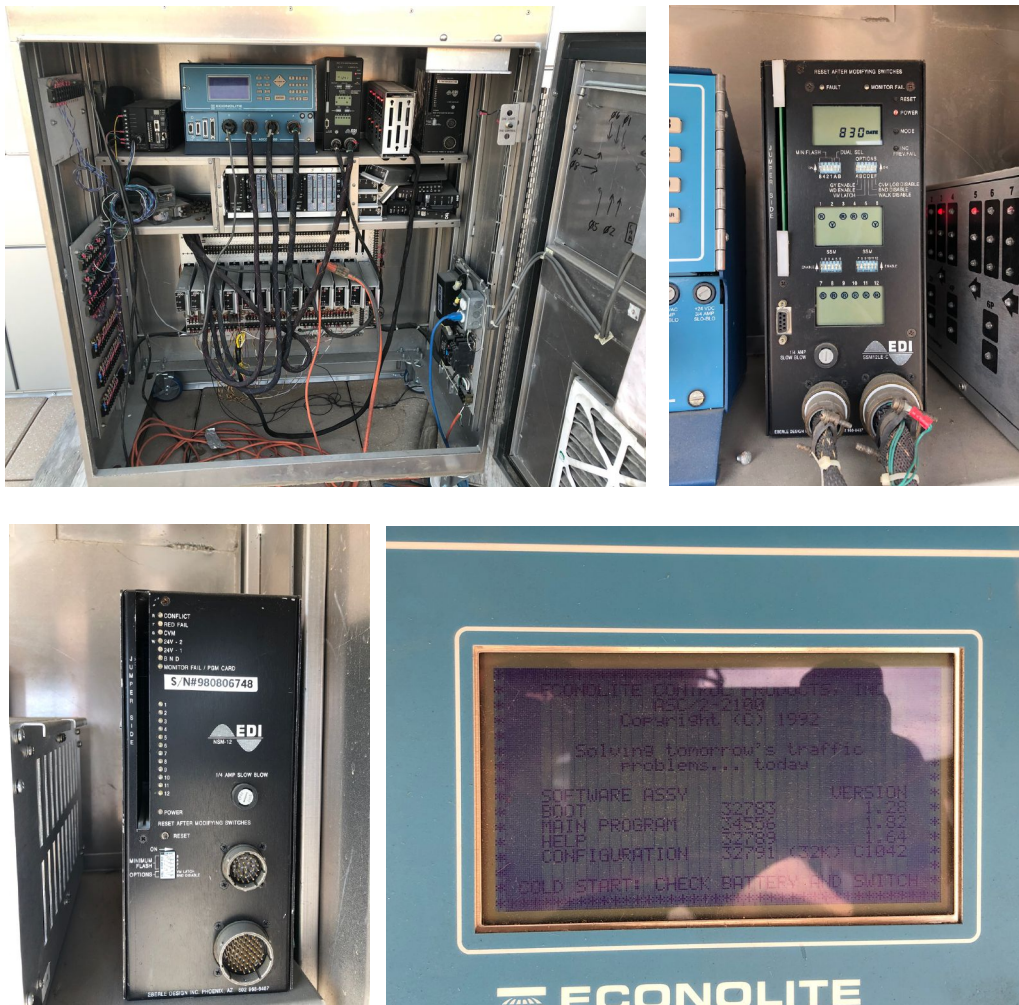
Figure 5 MMU equipment SSM-12LE(ip) signal monitor and NSM-12E were already installed inside the traffic control cabinet NEMA TS2 and have been testing our signals for 3 years on the roof.
