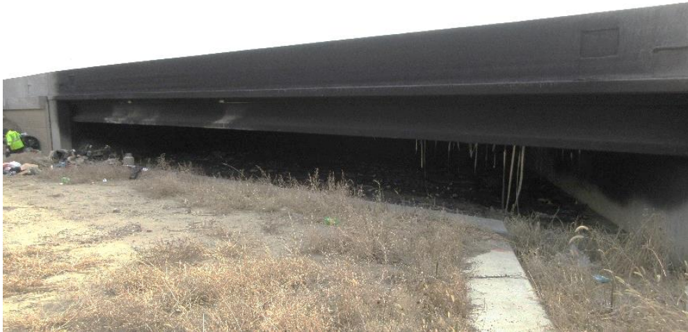
Figure 1 Bridge Fire on I-29 near Sioux City, IA
