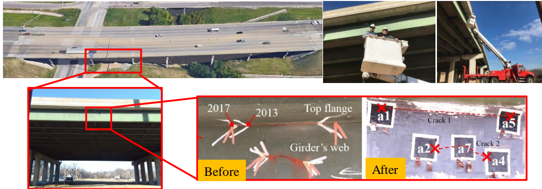
Figure 2: I-70 Bridge in Kansas with sensor network currently deployed
