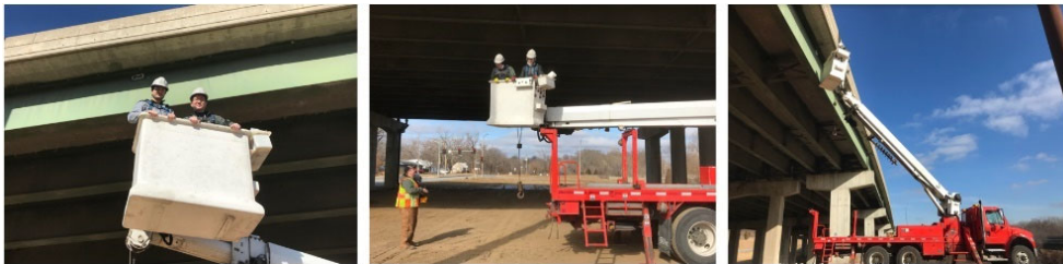
Figure 2. Field deployment of the monitoring system on a steel bridge.
