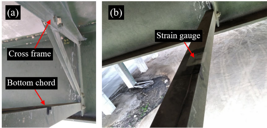
Figure 6. SEC installation on the interior side of the girder. (a) fatigue-susceptible region prior to the installation; and (b) SEC installation.
