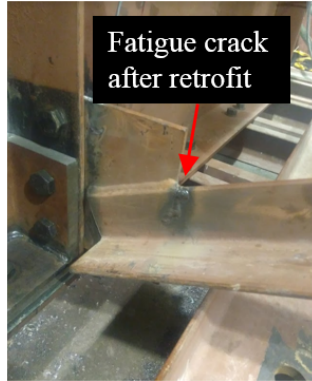
Figure 3. A fatigue crack was found at the diagonal member of the cross frame. The crack in the photo was later retrofitted by welding.
