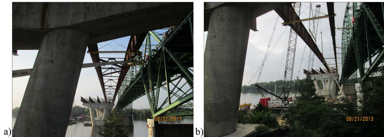
Figure 60. Field Erection of Girder Lines 1 and 2 Showing Successful Fit-Up of All Girders with a) View Under Pier and b) View Beside Pier (Photos provided by H. Pate, Tennessee Department of Transportation)
