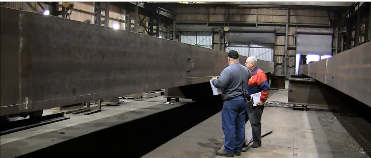
Figure 57. TDOT State Laydown Inspection of Girder Pair for BRIDGE VAS Detailed Splice Plates
