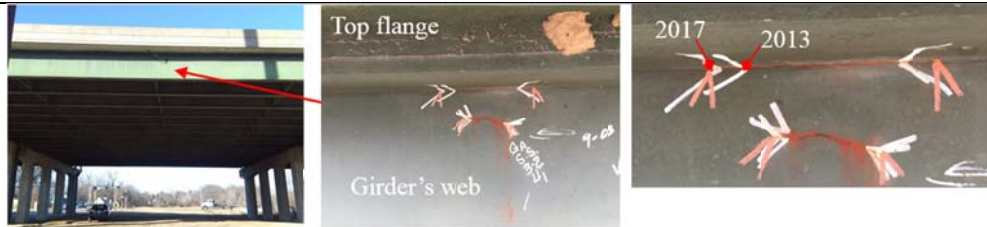
Figure 7. Detail views of the fatigue-susceptible region prior to sensor installation.
