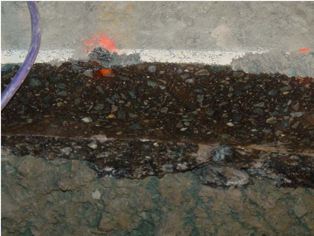
Figure 44. Cross section of the asphalt concrete showing asphalt material filling ruts created by construction traffic.
