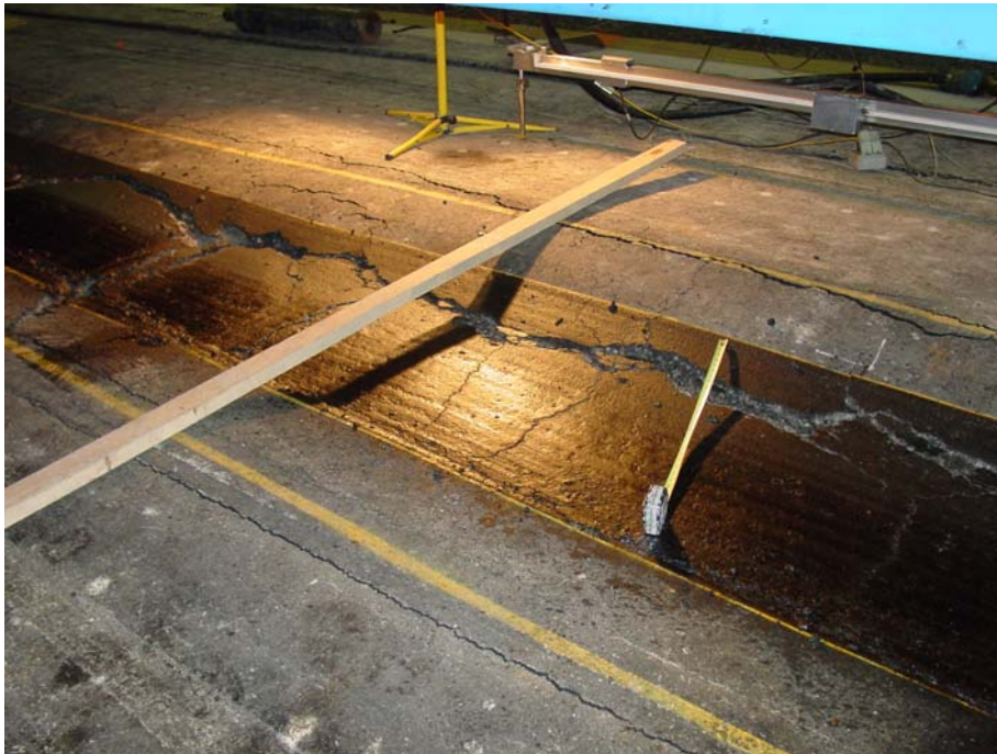
Figure 36. Pavement rutting and cracking at the end of HVS traffic on Test Window 5.
