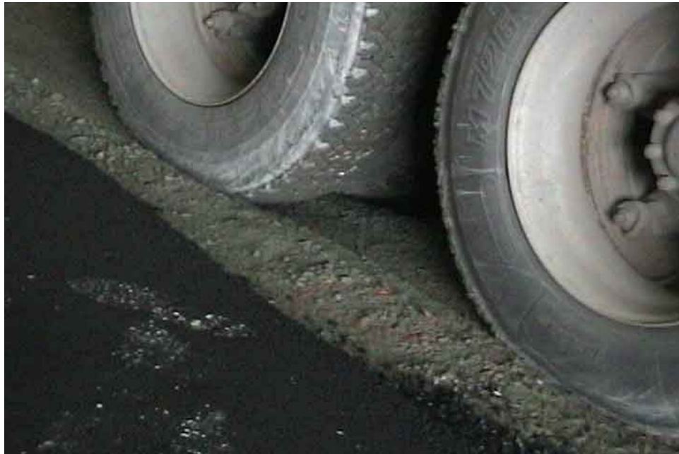
Figure 48. Ruts observed on top of the base course during the paving operation.
