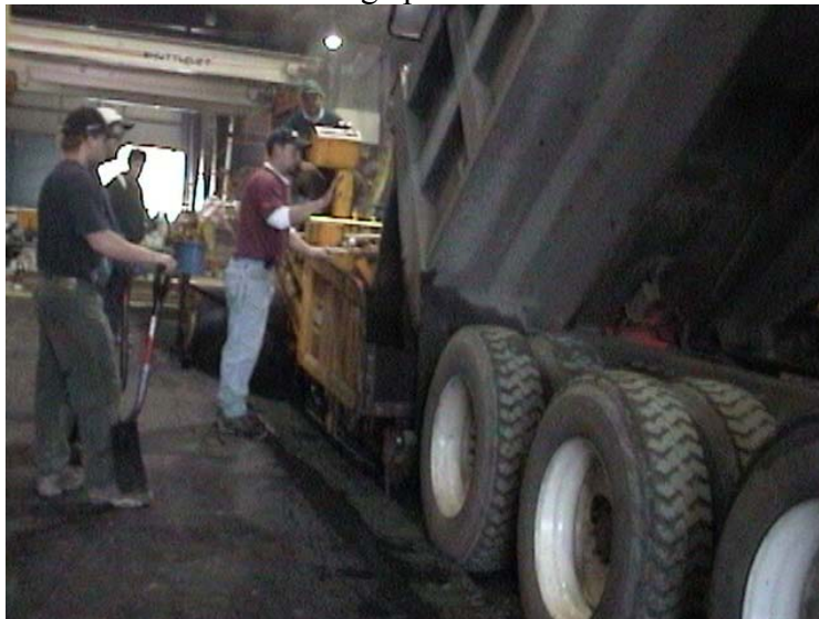
Figure 9. Construction loads caused significant ruts during the asphalt paving operation.
