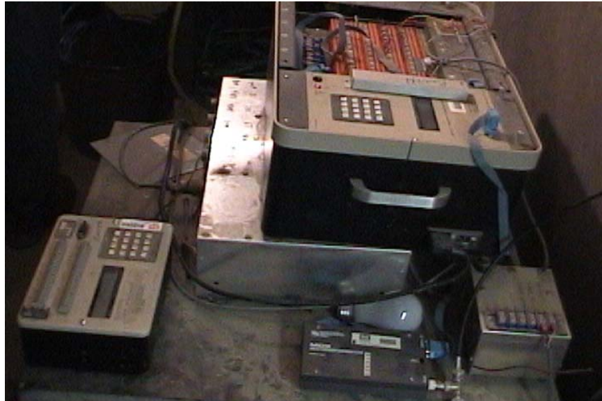
Figure 25. Data loggers used to measure and record moisture and temperature data.
