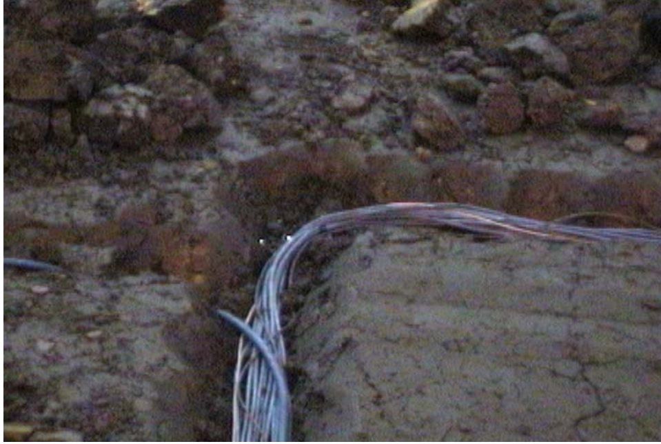
Figure 10. Sensor wires were routed toward the instrumentation tunnel.
