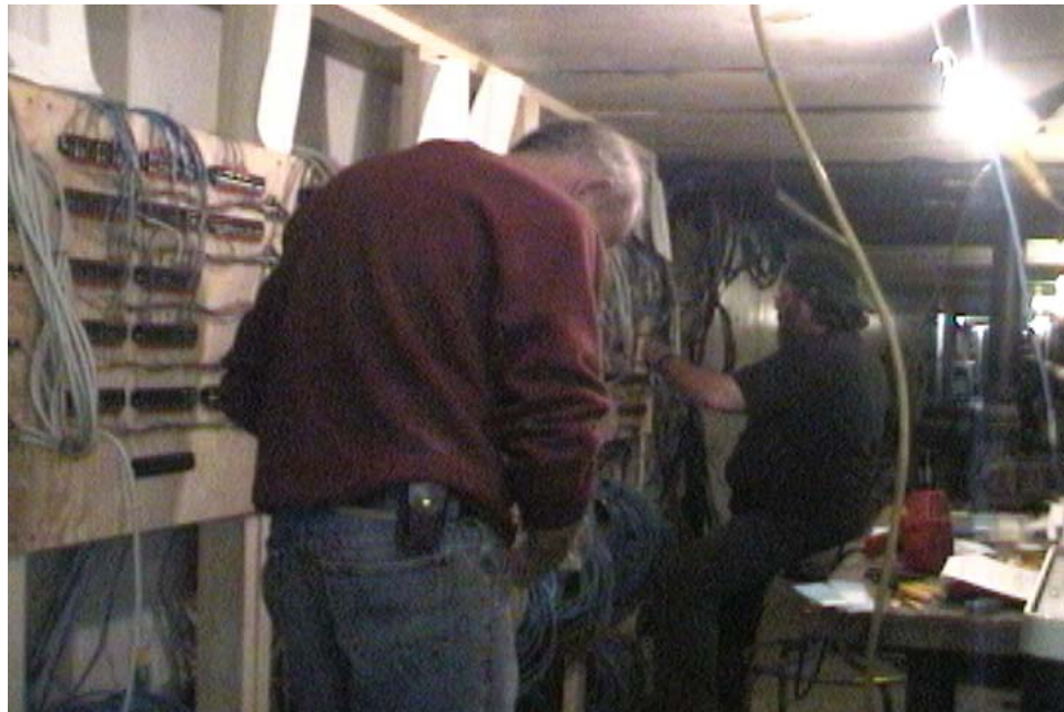
Figure 11. Sensor wire connections in the instrumentation tunnel.
