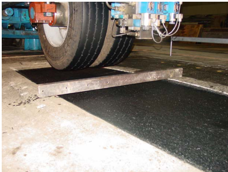
Figure 45. Soft spot and premature rutting in Test Window 711c6.
