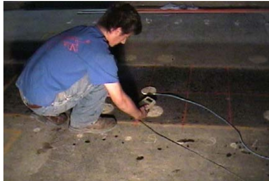
Figure 16. Measuring displacement between the AC surface and the top of the base course.
