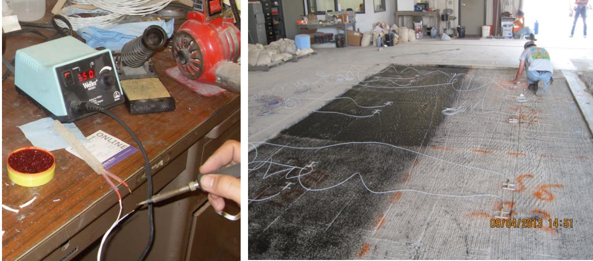
Figure 4.4: (a) Soldering New Lead Wires onto Strain Gages, (b) Installing Strain Gages after Tack is Applied
