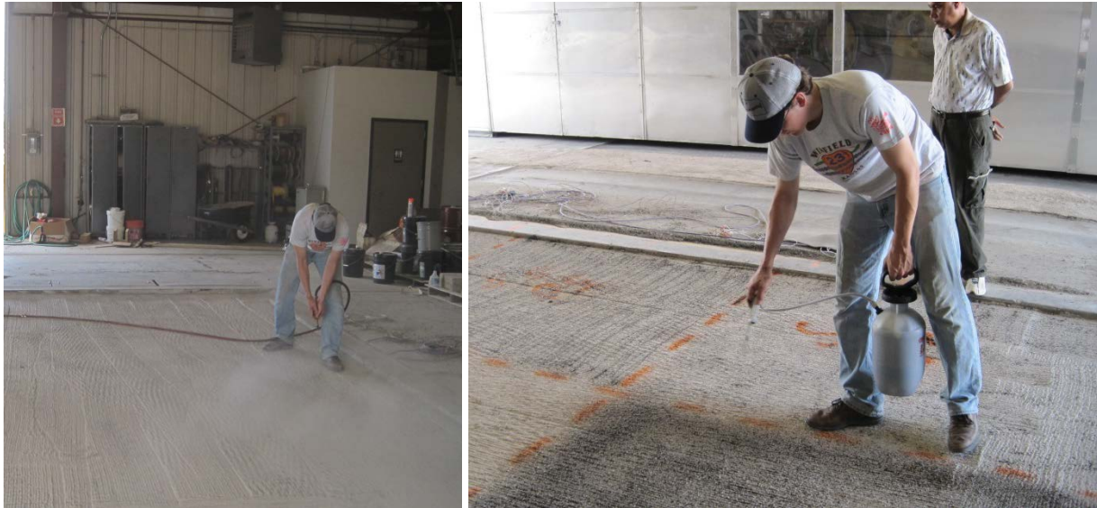
Figure 4.3: (a) Cleaning Surface with Compressed Air, (b) Applying Tack with Hand Sprayer
