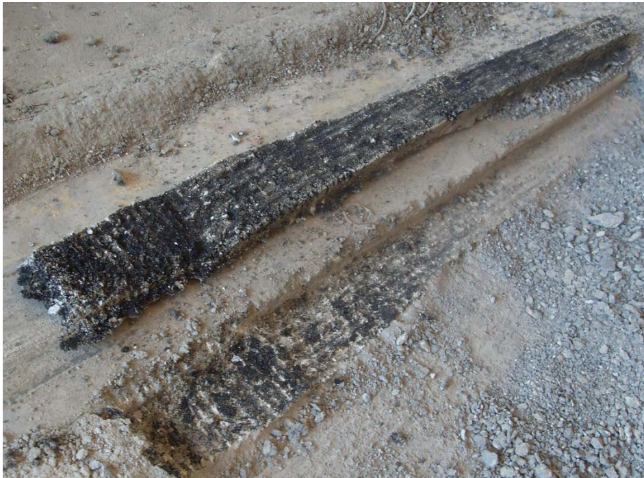
Figure 5.26: Edge of SE Section Easily Debonded during Milling
