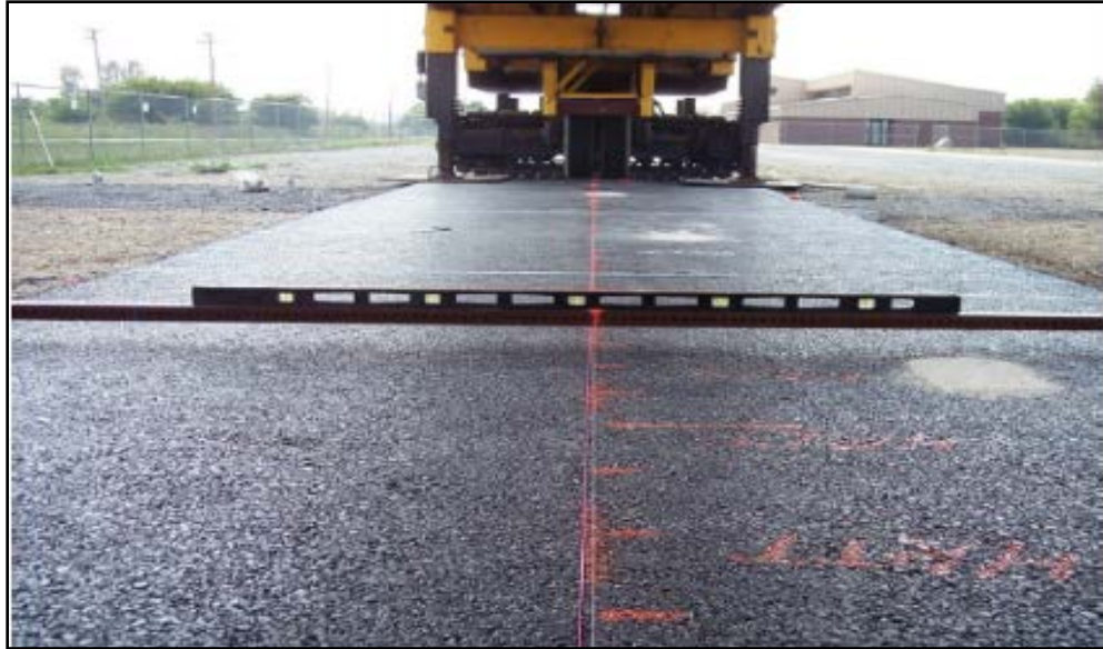
Figure 2.5: Surface Profile Measurements after APT Loading Source: Leng et al. (2009)
