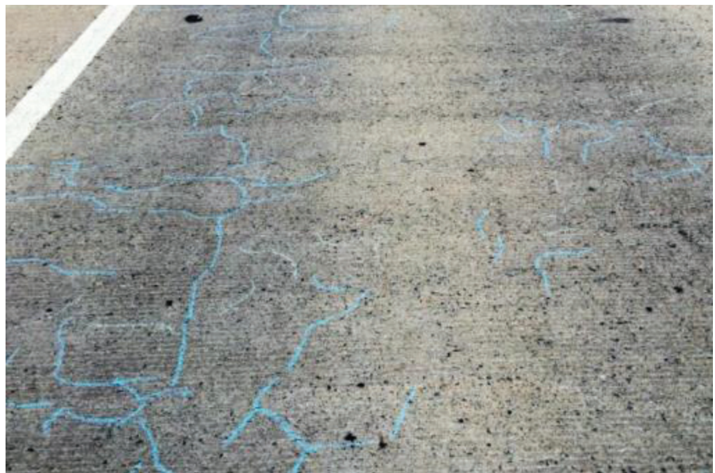
Map Cracks and Discolored
