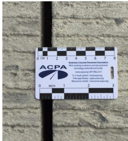
Activated joint (Approx. 0.5-in wide)
