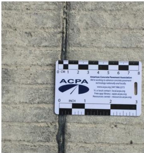
Un-activated joint (Approx. 0.25-in wide)
