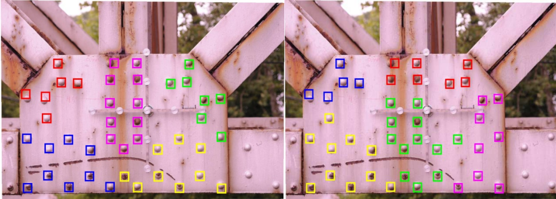
Figure 3.11: Gusset plate with loosely arranged fasteners. Fasteners grouped using k-means on the left and complete link Hierarchical clustering in the right. (k-means clustering performed better)
