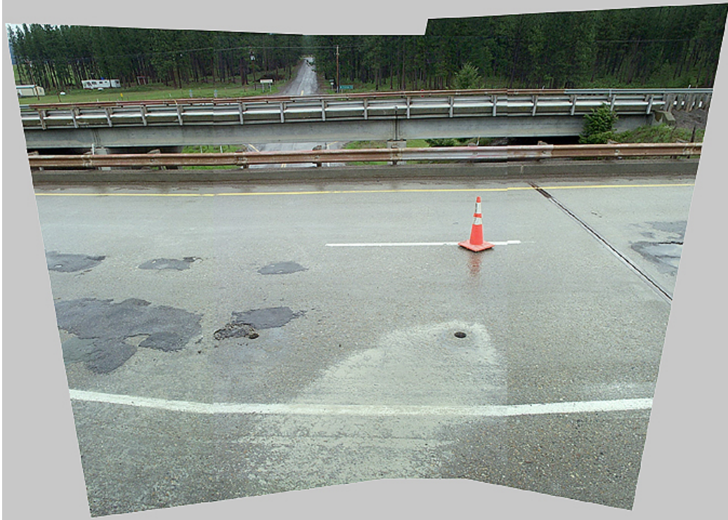
Figure 1: EB I-90 Tarkio interchange bridge deck after coring.
