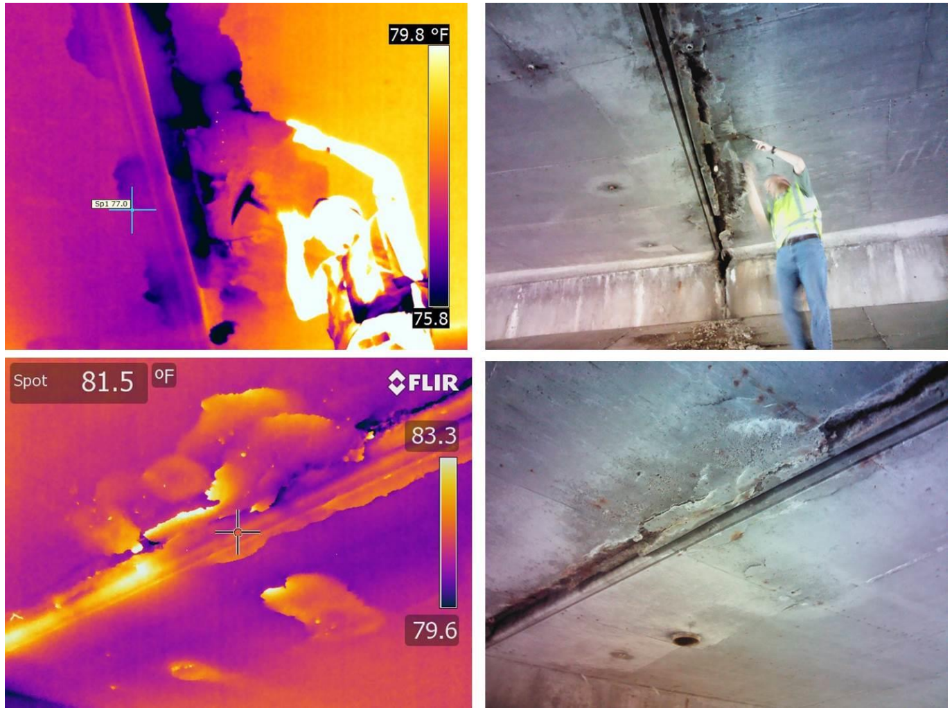
Figure 18. Thermal images showing damage along a longitudinal joint in a 159 ft wide slab bridge.
