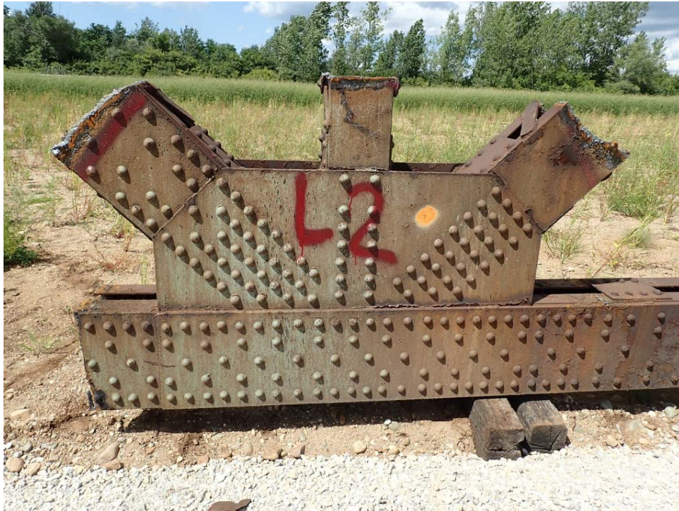
Gusset plate from CSX RR bridge in Philadelphia
