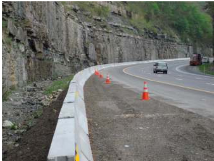
Figure 55. Location of I-24 scans showing ditch and highway (upper slopes not visible) (Photo courtesy of TDOT).
