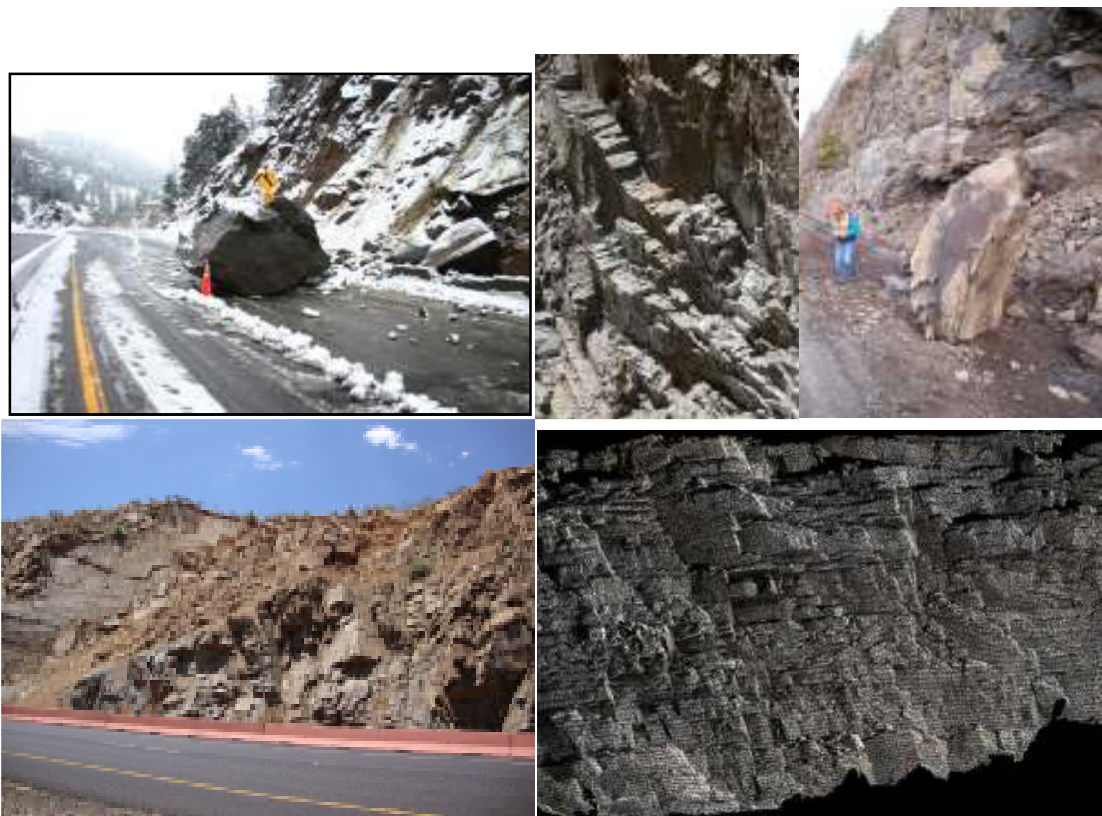
Figure 6. Images showing geotechnical issues associated with some of the pooled fund sites: top row, left to right, rockfall at one Colorado site, toppling at the California site, and rockfall at the Arizona site. Bottom left shows wedge failure at the Texas site, and bottom right shows overhangs at the New York site (Photos courtesy of CDOT).
