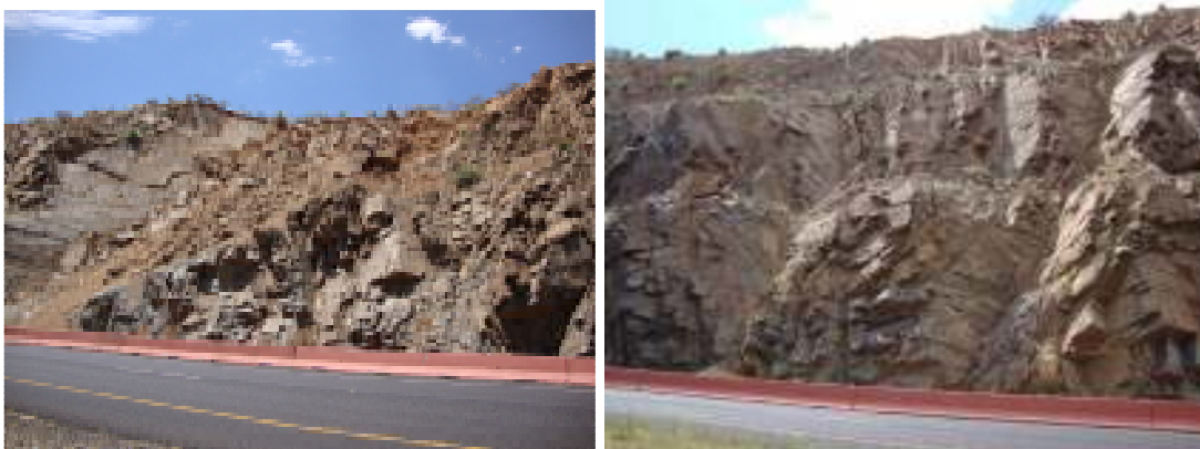
Figure 68. Wedge failures at the Texas site formed by discontinuity Sets 1 and 4 (see Figure 66b and Table 34).
