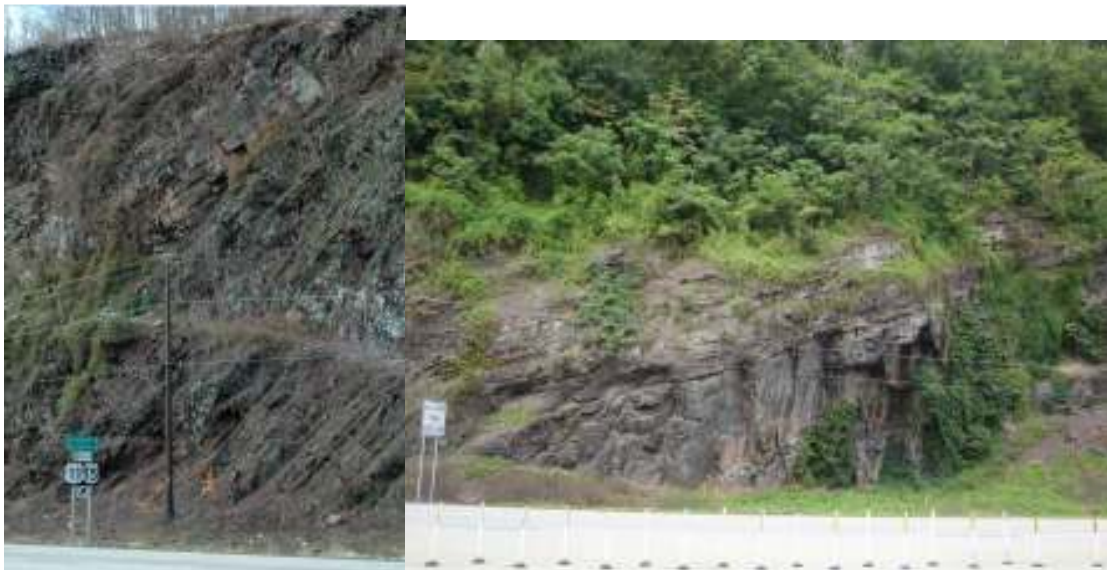
Figure 48. Left, a portion of the South Area scan, and at right, a portion of the North Area scan.
