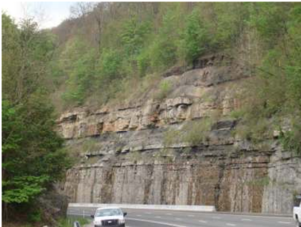
Figure 54. View of the highway cut on Interstate 24 westbound (Photo courtesy of TDOT).
