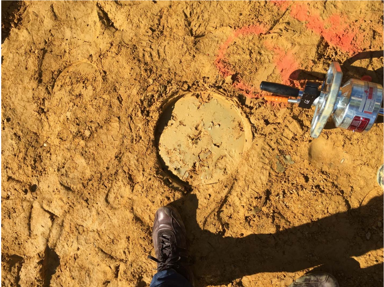
Figure 24. Excessive Permanent deformation observed at sections 5-10: SC soil (Clayey Sand)
