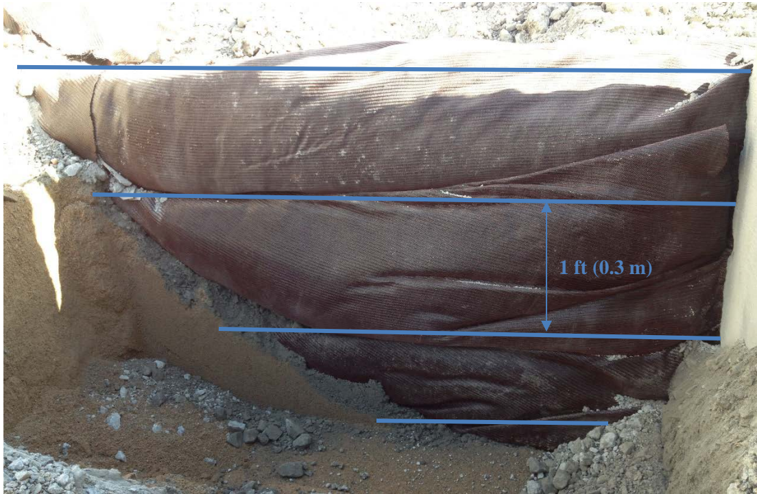
Figure 5. Geotextile fabric layer folds along the front of the backfill, shown by removing the west transverse wingwall after testing.
