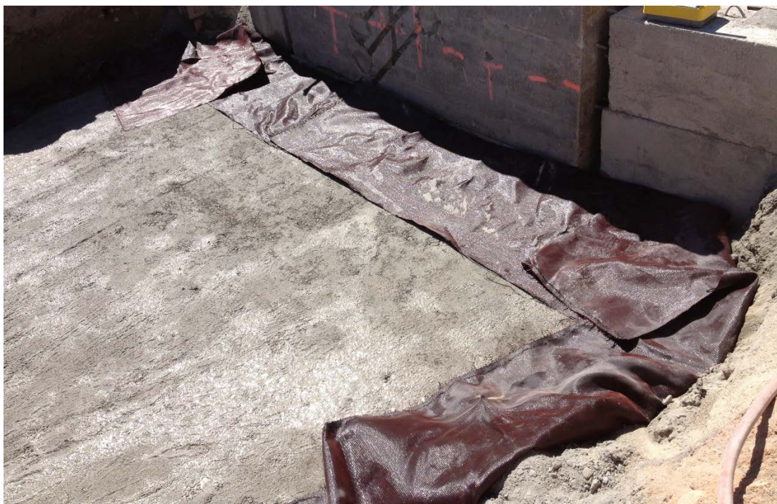
Figure 4. Fabric overlap of 3 ft (0.91m) between GRS layers, 0° test. Pictured is the top of a 1-ft (0.30-m) gravel layer before the next pieces of fabric were placed for the next layer.
