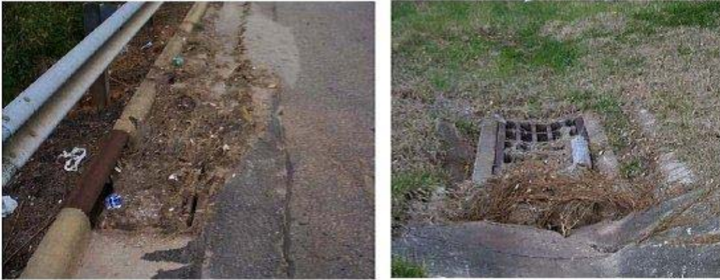
Figure A.6. Inlets blocked.
