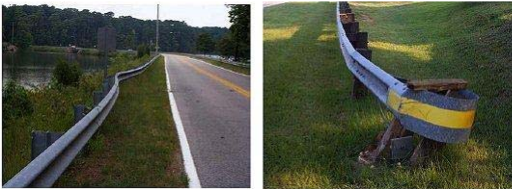
Figure A.7. Damaged barriers.
