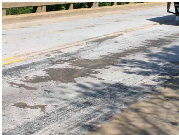
Figure 4.3. Patched concrete deck of bridge.
