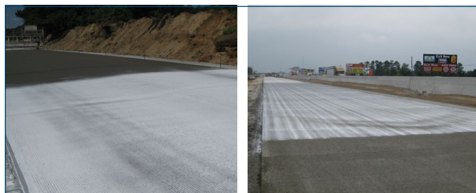
Figure 58. Poor curing practice
