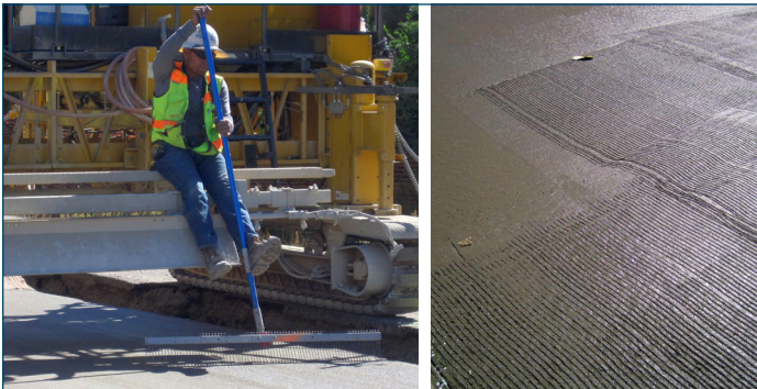
Figure 17. Manual longitudinal tining leading to undesirable texture variability (photo courtesy of Jim Grove)
