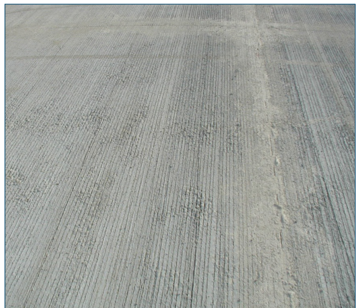
Figure 14. Variability in tined texture due to mix segregation/consistency problems
