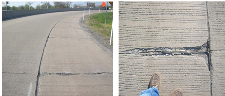
Fig. 1. Field observation showing damage in pavement joints
