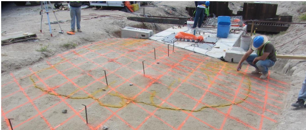
Figure 7-13: Completely developed failure wedge for the 30° test
