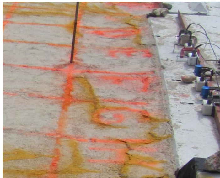
Figure 7-10: Transverse compression cracks at test completion
