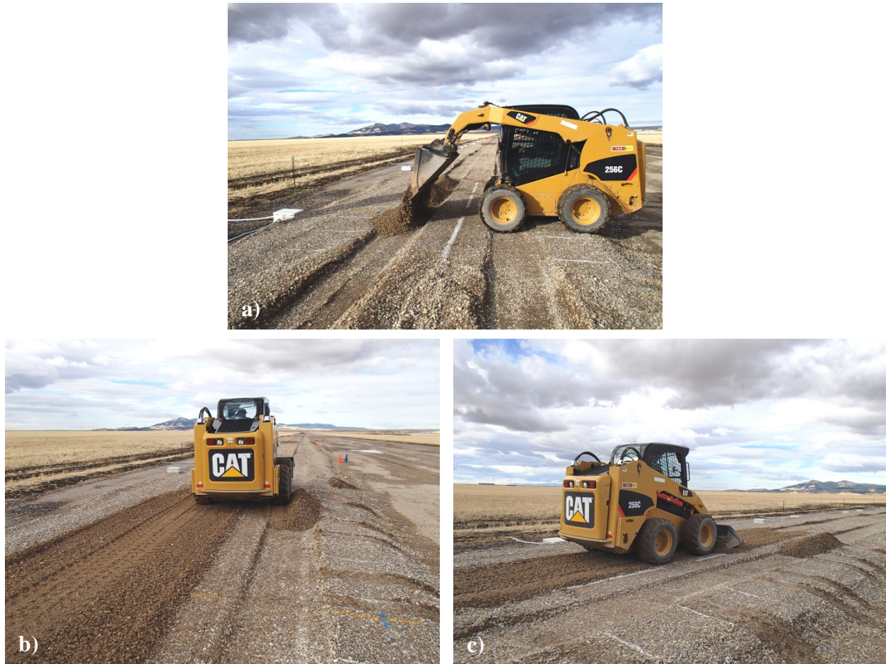
Figure 43: Rut repair: a) adding gravel to the rutted area, b) compacting the new gravel with the skid-steer tractor, and c) final smoothing.
