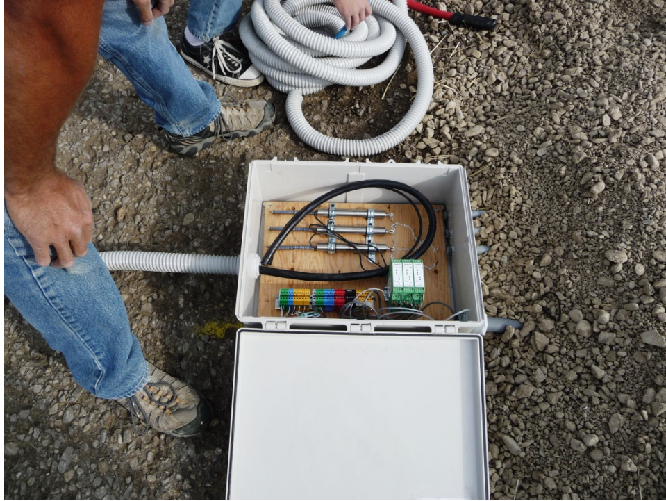
Figure 31. Instrumentation enclosure mounted to pavement.
