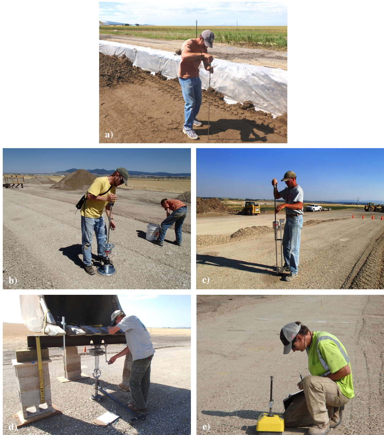
Figure 8. Construction quality measuring devices: a) vane shear, b) LWD, c) DCP, d) in-field CBR, and e) nuclear density.
