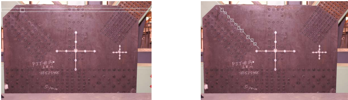
Figure 1. (Left) Step 1: Bolts are detected by scanning the bolt detector (the window marked white) across the image in raster scan. The detector identifies the locations and sizes of candidates that are likely to be bolts in the image. (Right) Step 2: The detected candidates can be grouped into clusters based on their collinearity. The figure shows one such cluster forming a straight line, which could help: (i) Estimate that one bolt detection is missing; (ii) Correct locations and sizes of the detected bolts.
