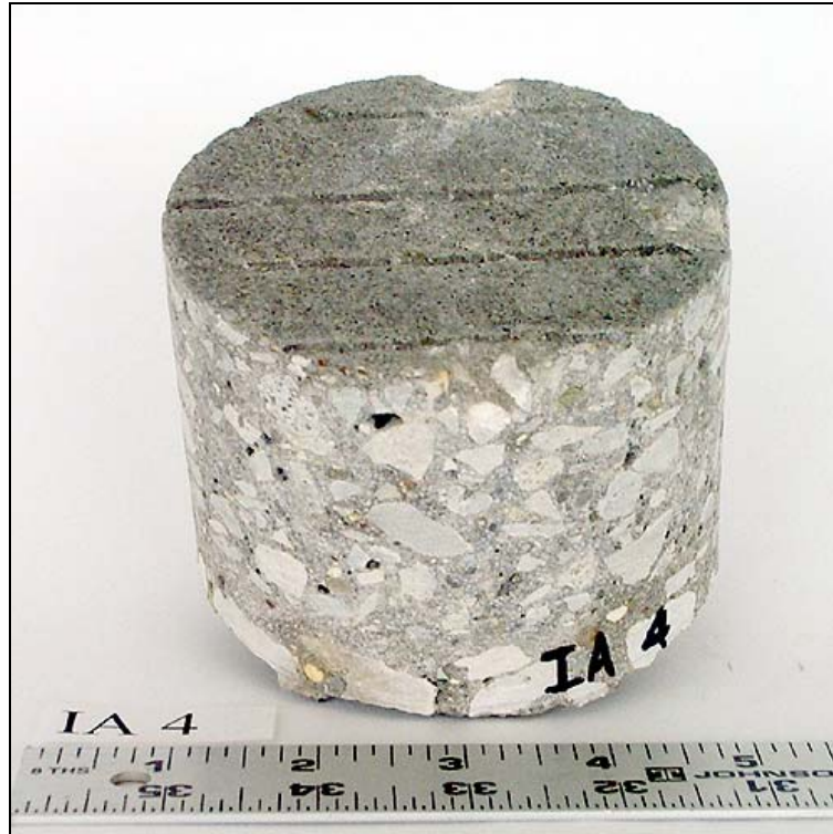
Figure 3.8. Core as received from Iowa site, without surface crack, (IA_04).
