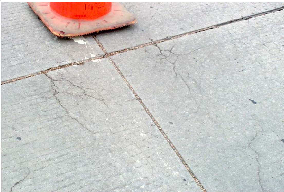
Figure 3.21. Photograph of cracks in pavement at Colorado site.
