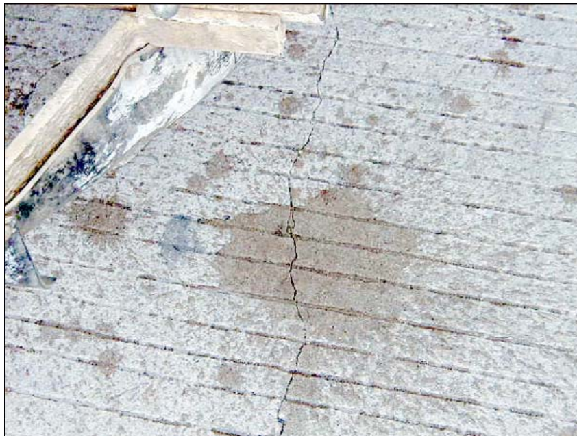
Figure 3.9. Photograph of crack at Iowa site.
