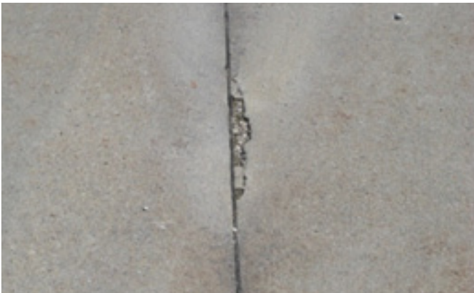
Figure 8. Water flow through joints from a high water table (bottom-up moisture); note staining on surface
