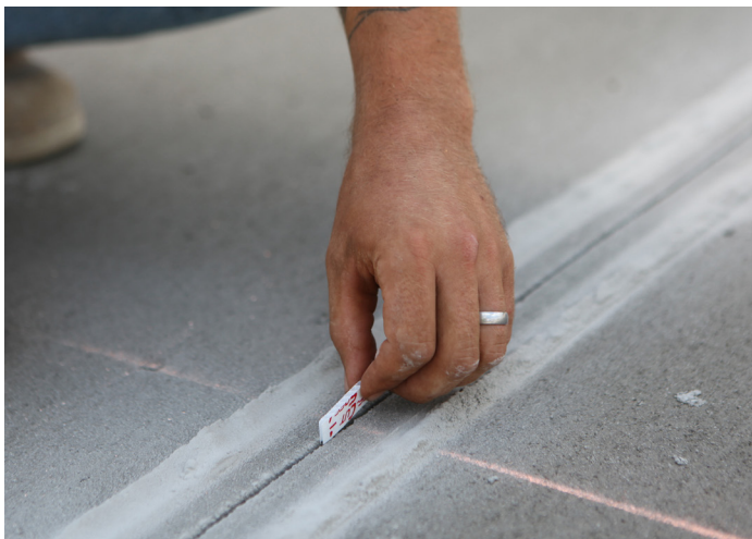
Figure 30. Using temporary joint spacers to protect and minimize damage due to early entry sawing (Source: Husqvarna)
