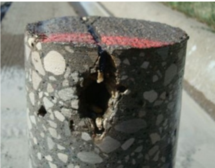
Figure 21. Joint deterioration evident below the joint sealant
