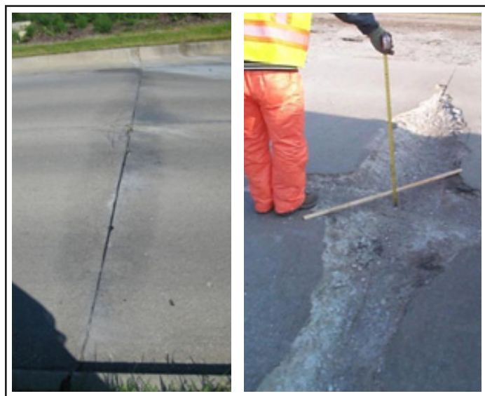
Figure 4. Evolution of joint deterioration from shadowing (left) to high severity (right)
