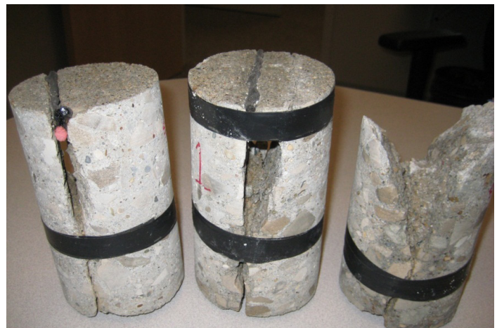
Figure 7. Three cores illustrating progression of distress from bottom-up moisture
