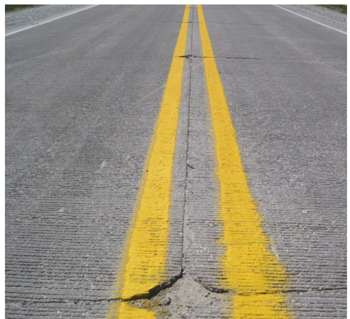
Figure 25. Damage starting at joint intersections
