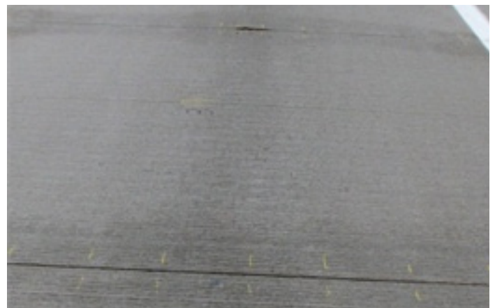
Figure 19. Shadowing at the joints, which is commonly followed by loss of material
