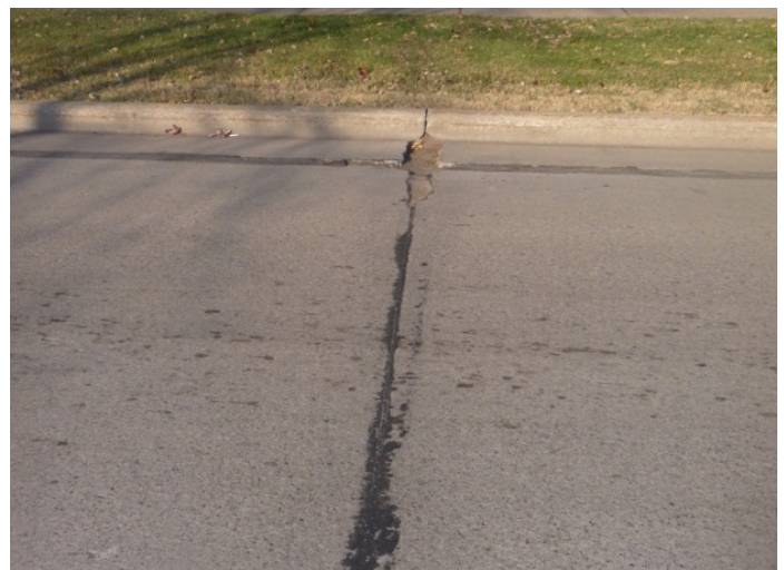
Figure 33. Failing transverse joint associated with poor drainage at gutter
