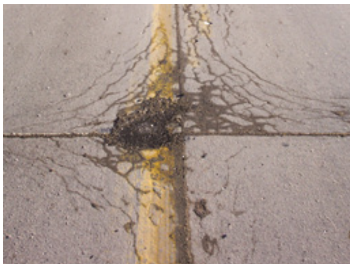
Figure 22. Deterioration due to D cracking
