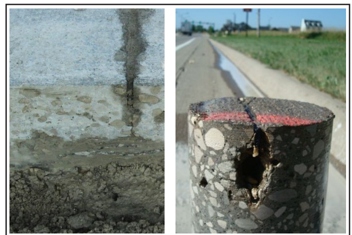
Figure 3. Saturated soils due to inadequate drainage and roadside irrigation (left) leading to joints showing frost damage (right) (Source: Snyder and Associates)
