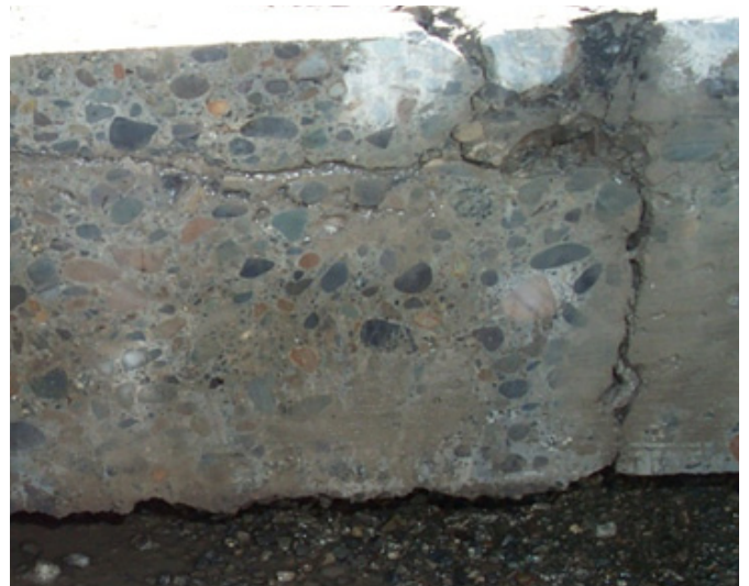
Figure 18. Example of delaminations spalling (Source: Washington State)
