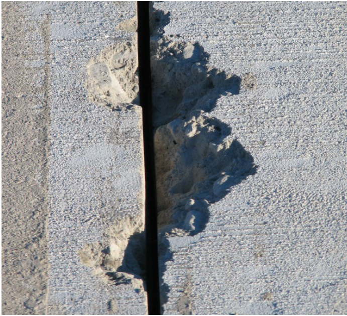
Figure 14. Raveling due to poor sawing practice (Source: Iowa Department of Transportation)
