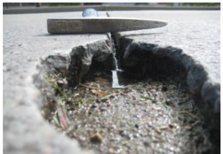
Figure 27. Example of a poorly draining pavement
