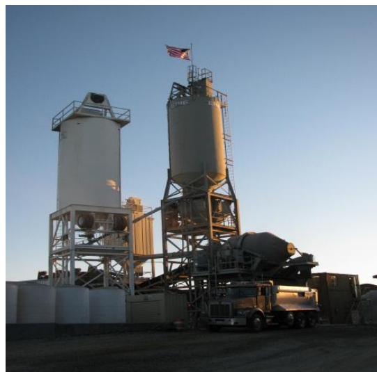
Figure 4. Central mix plant
