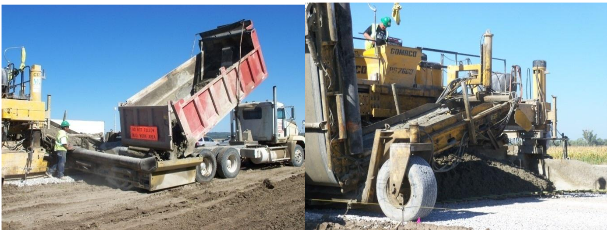
Figures 6 and 7. Concrete being dumped into a belt placer and spread by the placer
