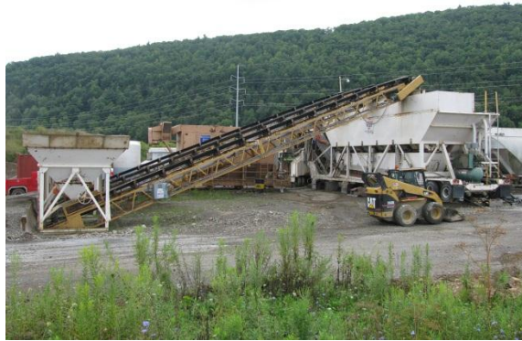
Figure 3. Concrete central mix plant
