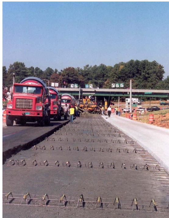
Figure 5-97: Dowels can be placed within acceptable tolerances, field measurement every day is critical
