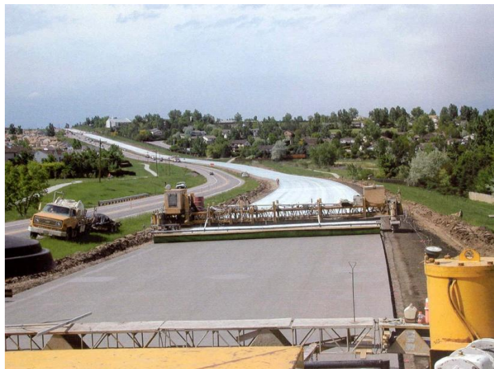
Figure 5-96: Curing of concrete pavements is critical; water cure eliminates built-in temperature gradients, high zero-stress temperature, and excessive shrinkage.
