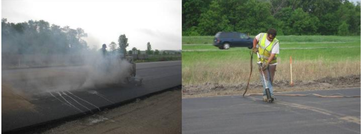
Figure 5-110. Sawing joints in the AC layer which correspond to the joints in the underlying PCC layer (left) and sealing the newly sawn joints (from Rao et al 2011)
