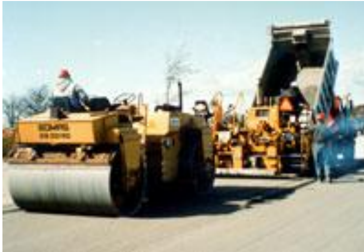
Figure 5-101: Typical RCC paving operation: dump truck unloads mix into an asphalt paver, a roller follows close behind to ensure adequate compaction (from Portland Cement Association, 2012).
