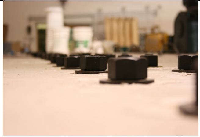
Fig. 2 A325 bolts connecting the deck to the girder top flanges to develop composite action
