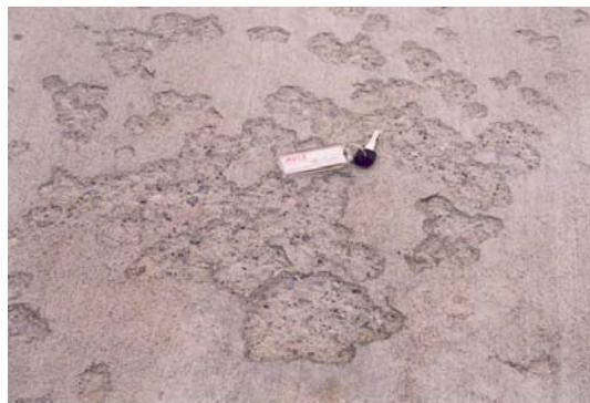
Figure 2. Example of salt-scaling damage.
