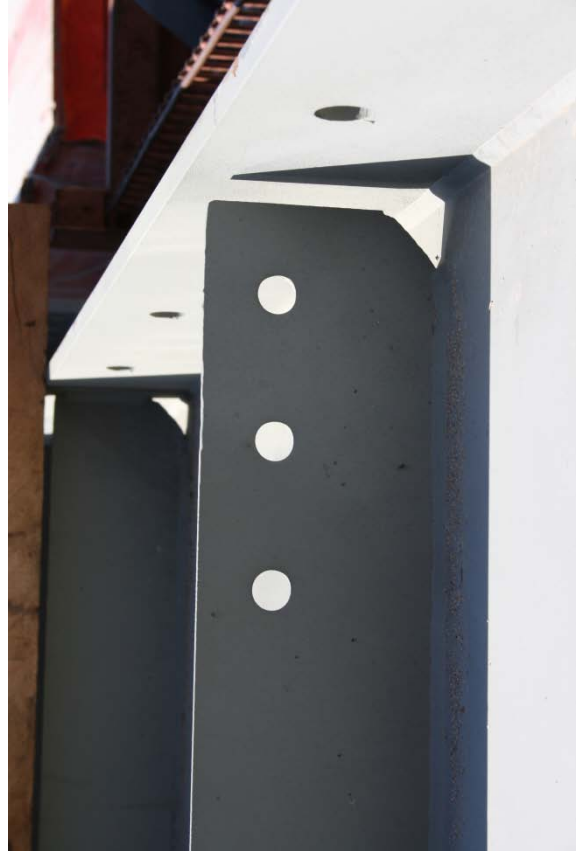
Fig. 2. View of web gap region in segment of test girder intended to develop fatigue failure
