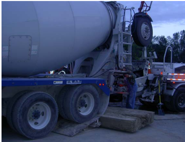
Fig. 5.4 – Example of a ramp used by ready-mix trucks to increase the chute angle and facilitate unloading the relatively low-slump LC-HPC.
