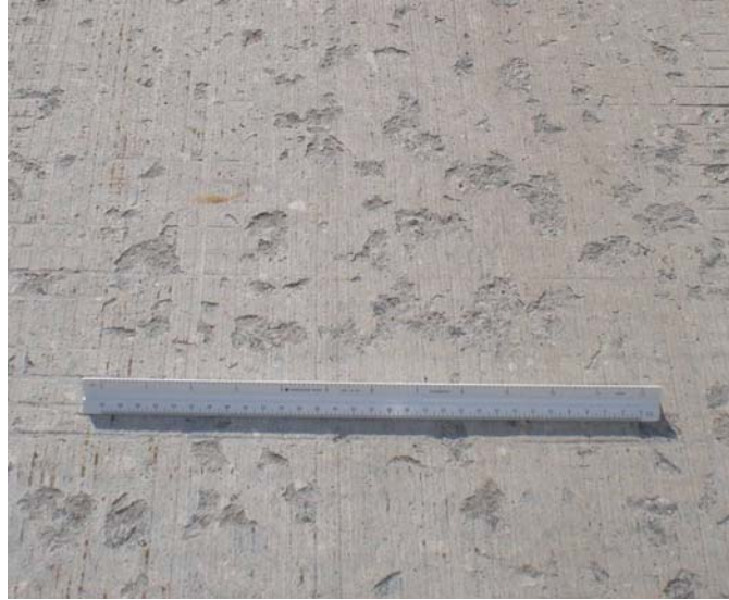
Fig. 5.6 – Typical scaling observed in the gutter areas of LC-HPC-2
