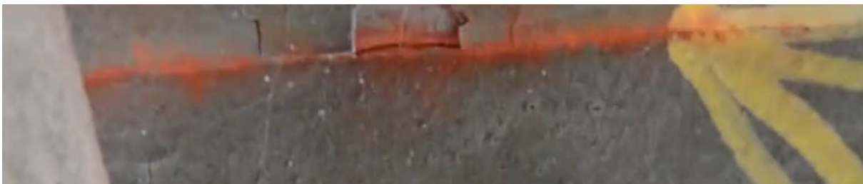
Figure 1. A video frame of fatigue crack after video stabilization and motion magnification
