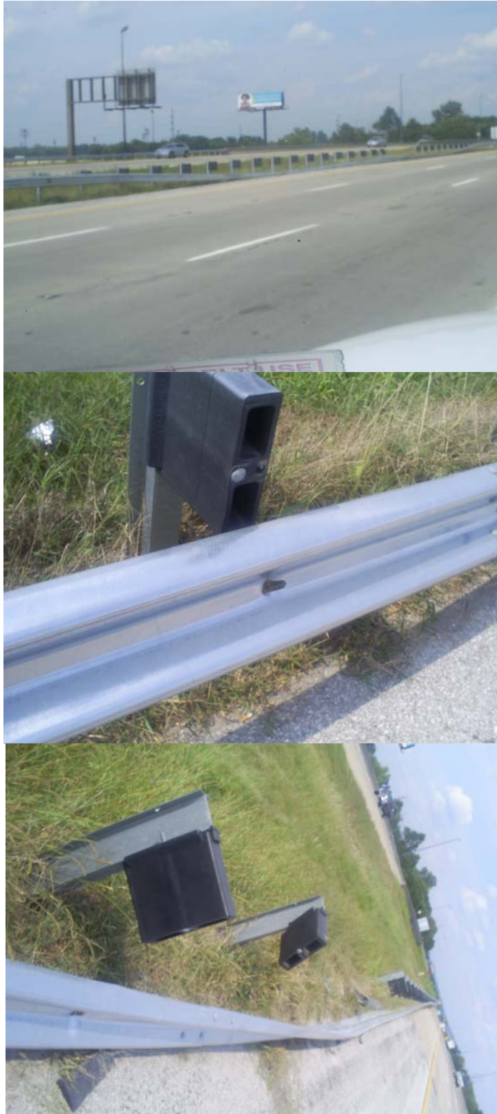
Figure 2. MGS Guardrail Damage
