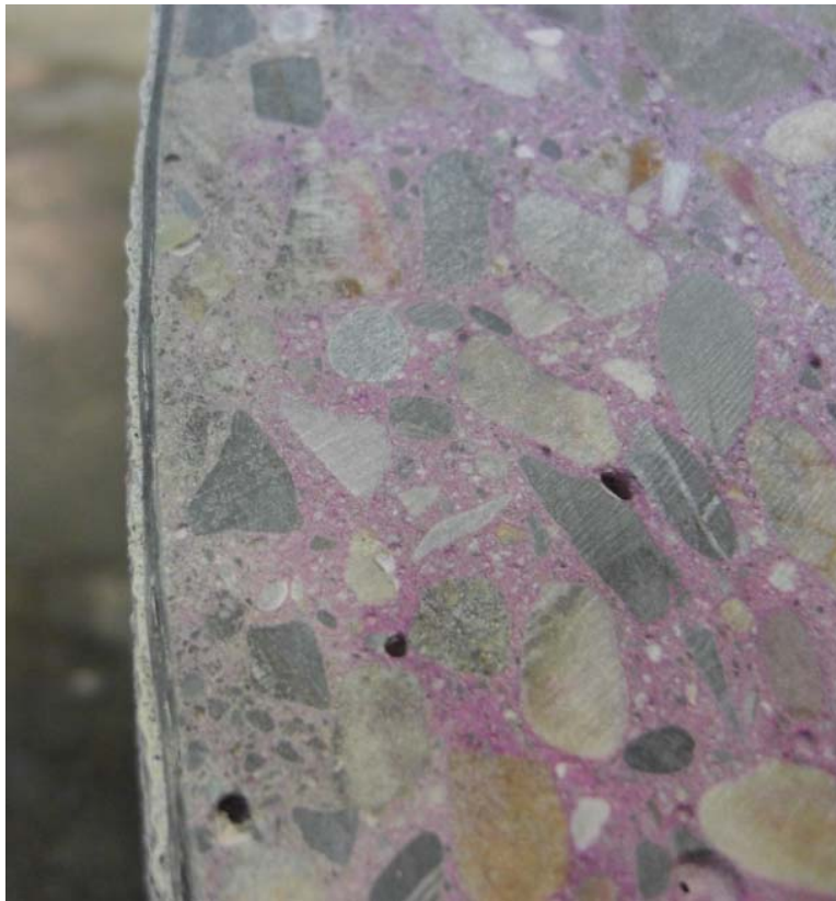
Figure 5. Concrete carbonation at perimeter of cut-off column section.
