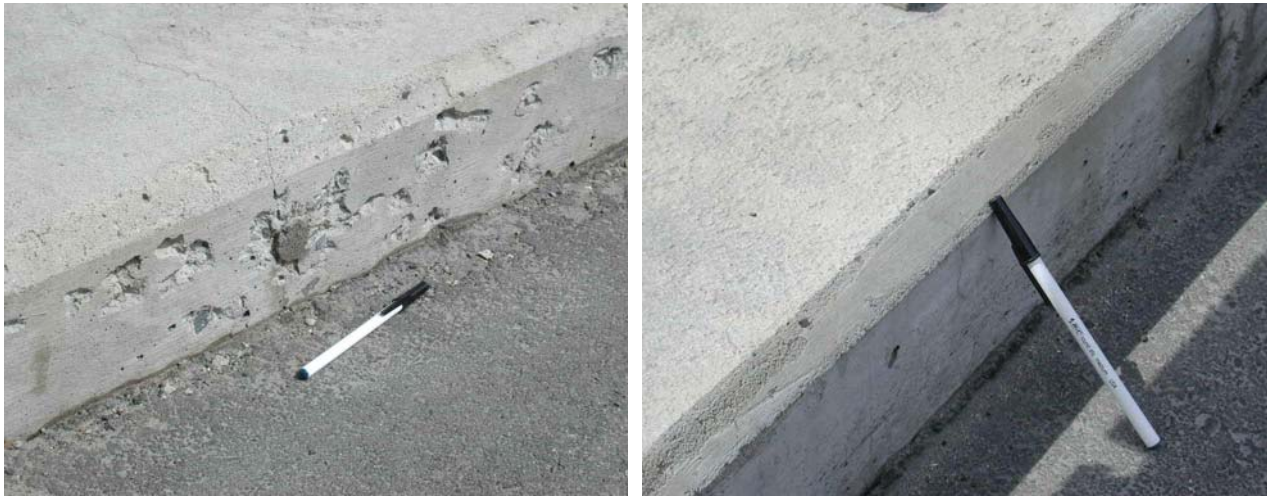
Figure 3. After two winters, the control concrete (left) is beginning to spall while the antifreeze concrete is unchanged.
