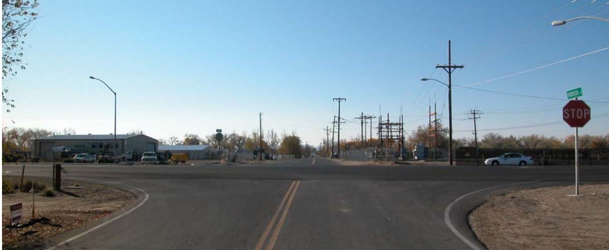
FIGURE 4-1 Business in the Southeast Quadrant (left) and an Electrical Transformer Station in the Southwest (right) Quadrant
