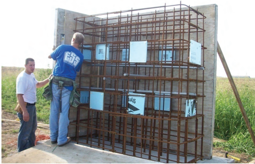
Figure 3.3 : Photograph of the test block during construction showing the targets mounted on the rebar cage.
