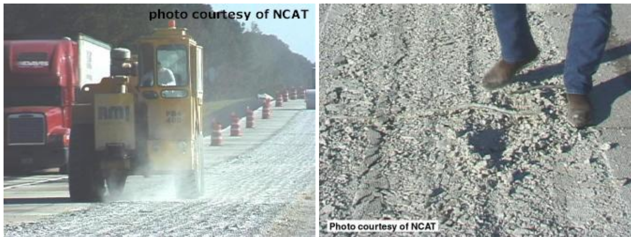
Figure 3.5. At left, resonant pavement breaker used to rubblize PCC pavement; at right, PCC pavement after rubblization with a resonant pavement breaker (WSDOT).
