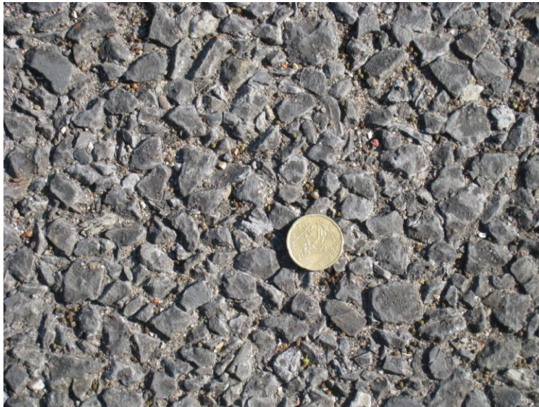
Figure 4.2. Close-up of the porous asphalt surface of the A12 motorway. Note fines infiltrating the porous asphalt surface on the edge of the traffic lane (SHRP2 2009).
