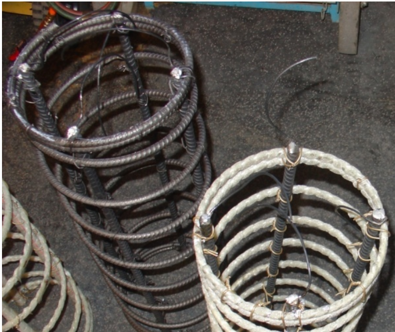
Figure 4. Wires attached to four vertical bars in the steel reinforcement at the top.
