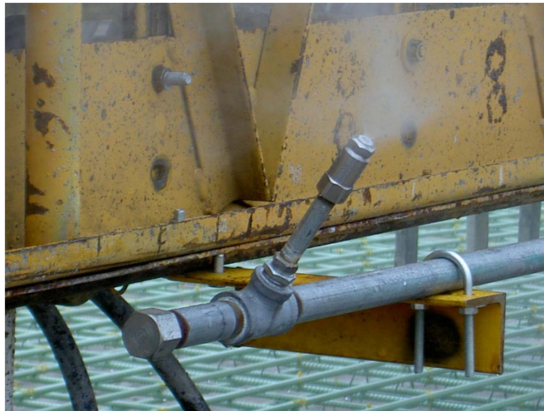
Fig. 5.25 Fogging equipment that worked well, producing fog and did not drip
