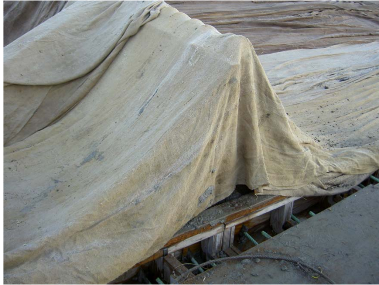
Fig. 5.10 Burlap draped over reinforcement without contact at the base
