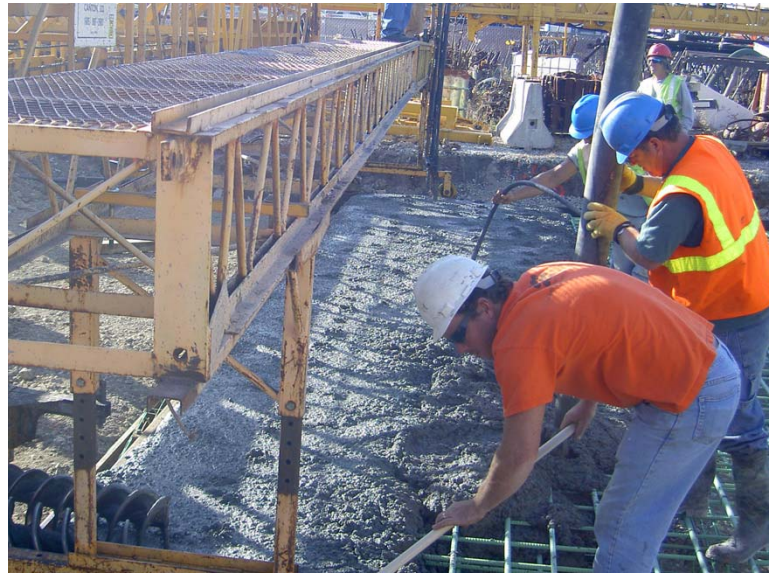
Fig. 5.39 Coarse aggregate particles above the concrete surface indicates concrete is underconsolidated and holes in the concrete from where vibrators were located, indicating that the vibrators were removed too quickly leaving no coarse aggregate at the insertion points
