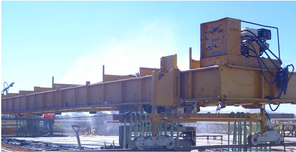
Fig. 5.20 Fog misting the air over the deck without depositing water onto the surface of the deck during a delay in concrete placement
