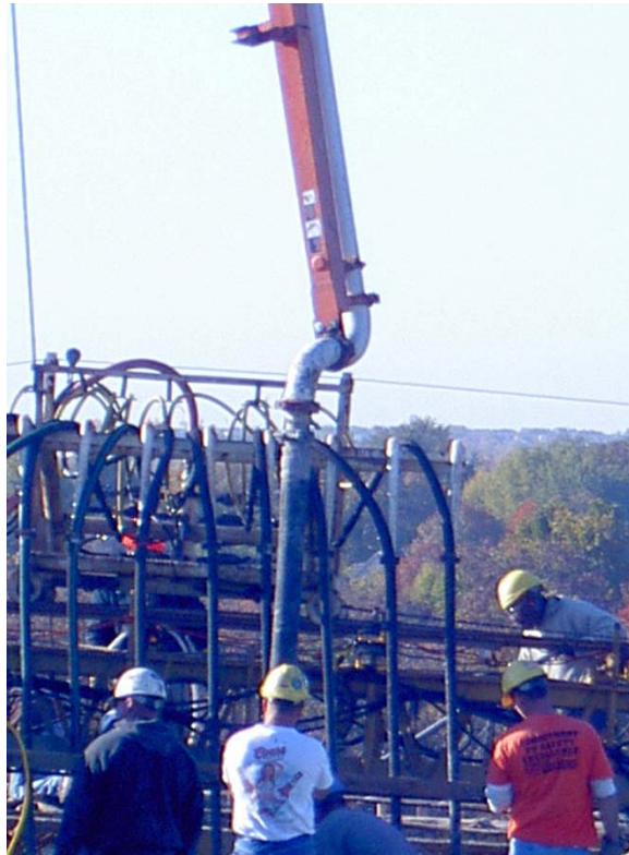
Fig. 5.32 (a) First pump did not have an air cuff
