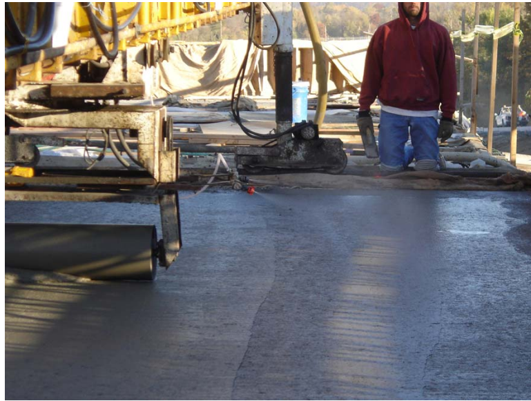
Fig. 5.7 Fogging system mounted on roller screed and spraying water onto the concrete surface – this practice increases the potential for cracking
