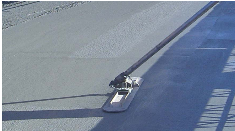
Fig. 5.42 The surface finish after the screed was acceptable and bullfloating was not necessary
