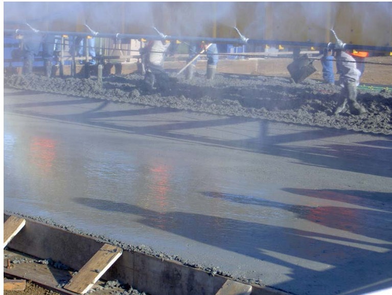
Fig 5.18. Excessive surface water deposited onto the deck by the fogging.
