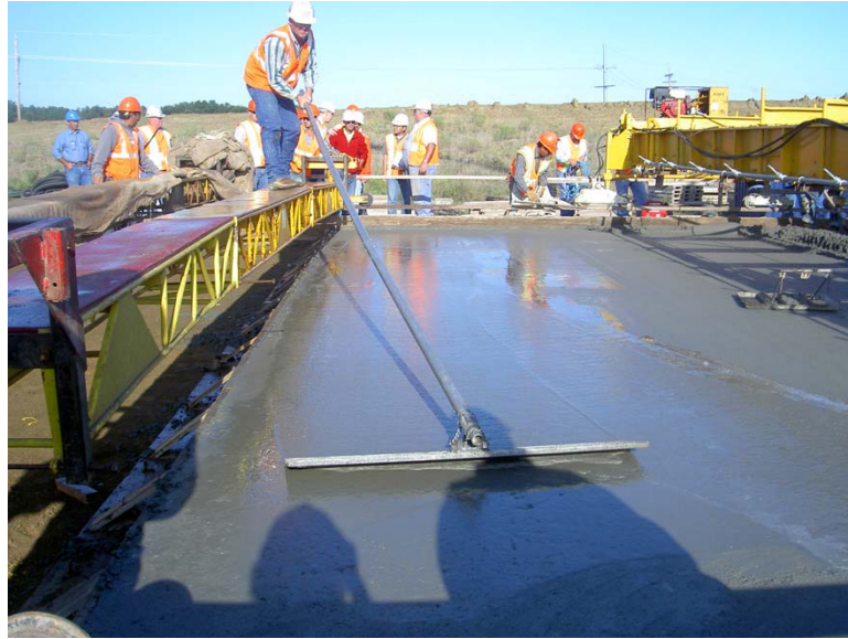
Fig. 5.19. Water from fogging used as finishing aid – increases the potential for cracking
