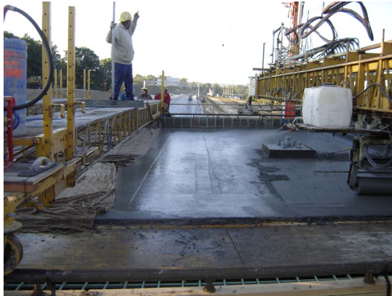
Fig. 5.2 Fogging system spraying water onto the deck surface, which was worked into the surface of the deck by the bullfloating operation – this practice increases the potential for cracking
