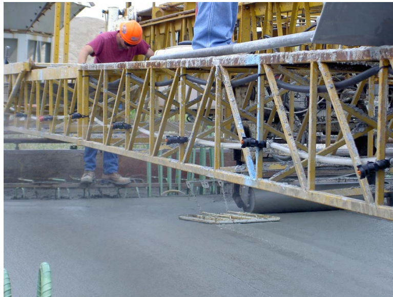
Fig. 5.1 Fogging system depositing excessive water on the deck surface
