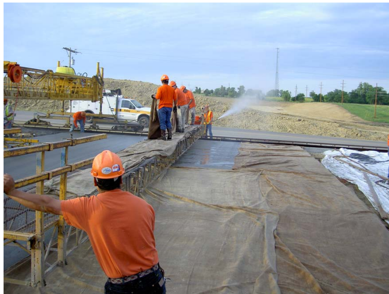
Fig. 5.12 Water ponding on deck surface due to hand fogging and burlap dripping on the surface. Using only one work bridge to place burlap is slow and did not meet the time requirements
