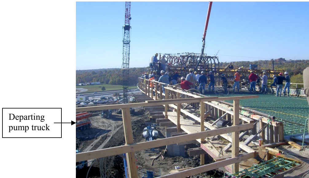
(d) Second pump used for last portion of the deck while the first pump is departing the site
