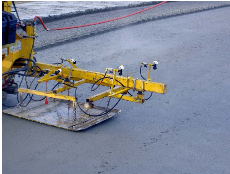
Fig. 5.11 Fogging equipment mounted in an undesirable location on the pan drag close to the deck surface
