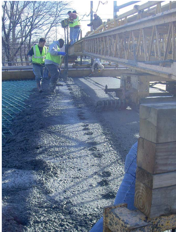
Fig. 5.40 Coarse aggregate particles and a consolidation lip at the locations of vibrator insertion indicate inadequate consolidation
