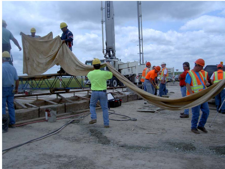
Fig. 5.26 Workers standing far from the slab does not accurately simulate conditions on the deck
