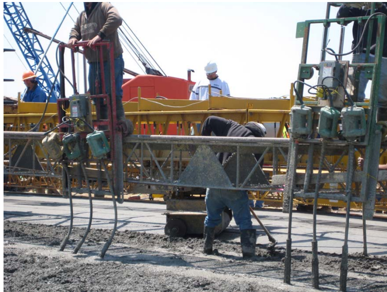
Fig. 5.38 Two sets of gang vibrators mounted on work bridge separate from finishing bridge with worker walking in consolidated concrete
