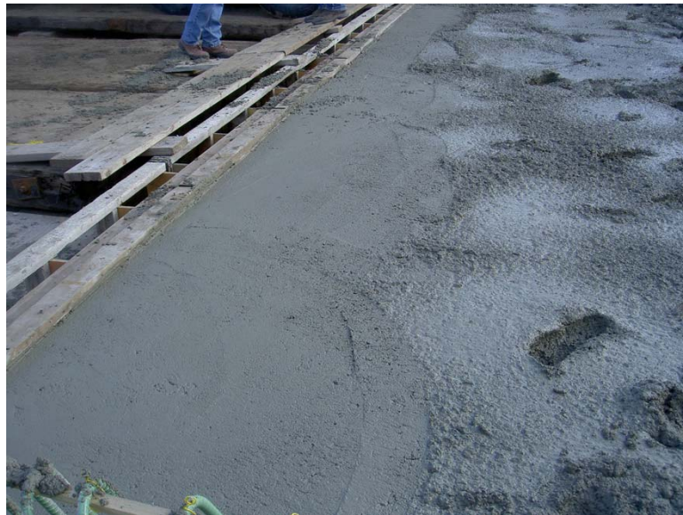
Fig. 5.28 Insertion points for hand vibration at the west end of LC-HPC-11 are farther apart than for the gang vibration.
