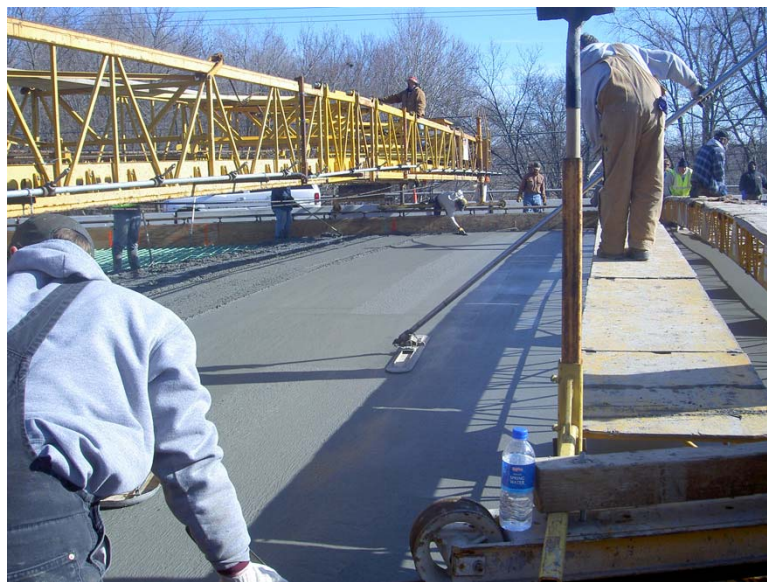
Fig. 5.41 Bullfloating performed perpendicular to finishing bridge is slower and causes delays in burlap placement.
