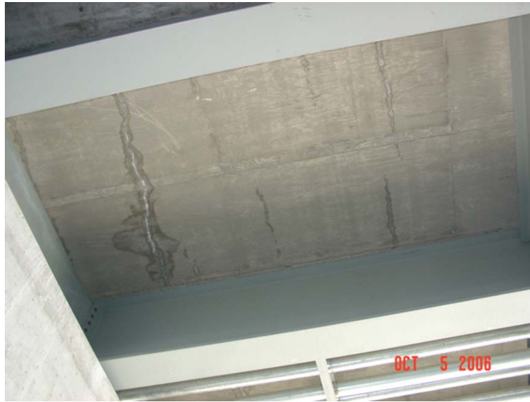
Fig. 5.14 Through-depth cracking on the underside of Control 7 deck.
