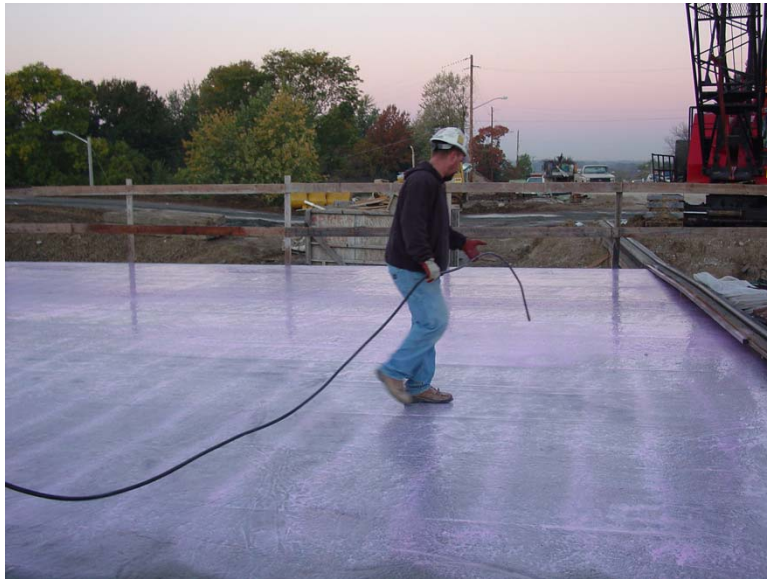
Fig. 5.4 (b) Application of the second coat – worker damaging the first coat by walking on it
