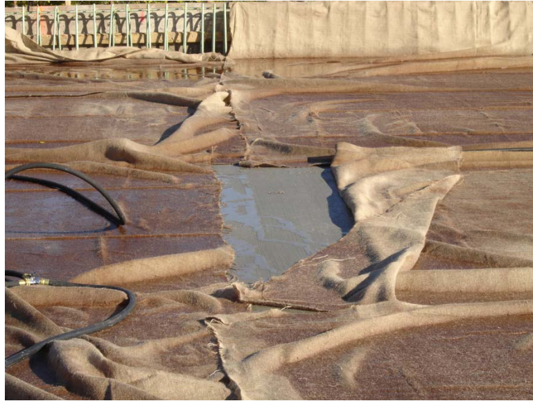
Fig. 5.35 Burlap that was not overlapped sufficiently, so pieces were dislocated by the wind leaving concrete exposed
