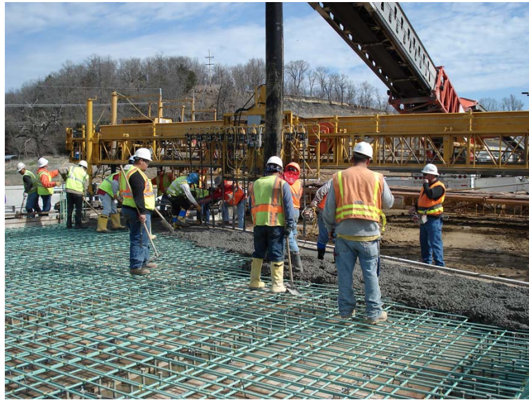
Fig. 5.21 (a) For the north portion of deck the drop was approximately 6.1 m (20 ft)
