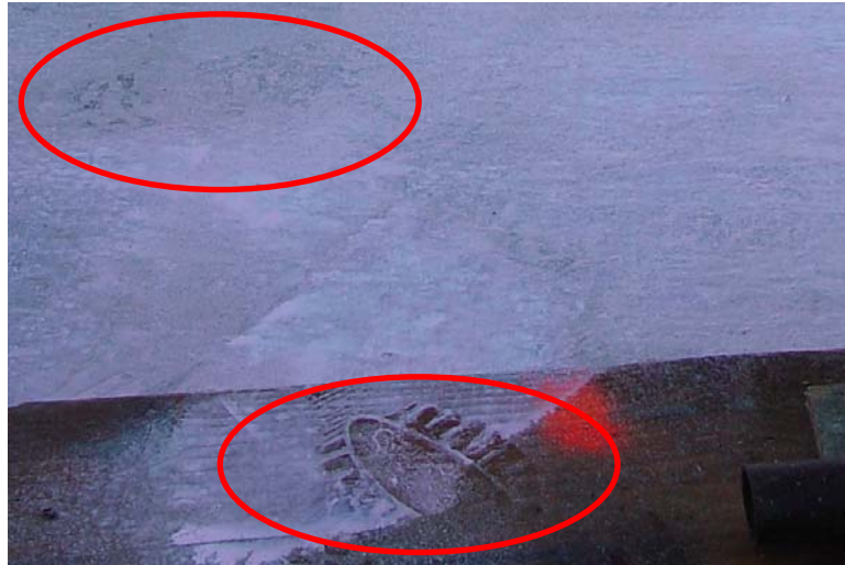
(c) Damage to wet curing membrane due to footprints
