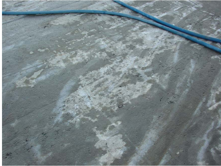
Fig. 5.6 Divots observed in the deck surface
