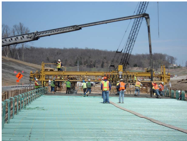
Fig. 5.21 (b) For the center portion of deck the drop was approximately 11 m (36 ft)
